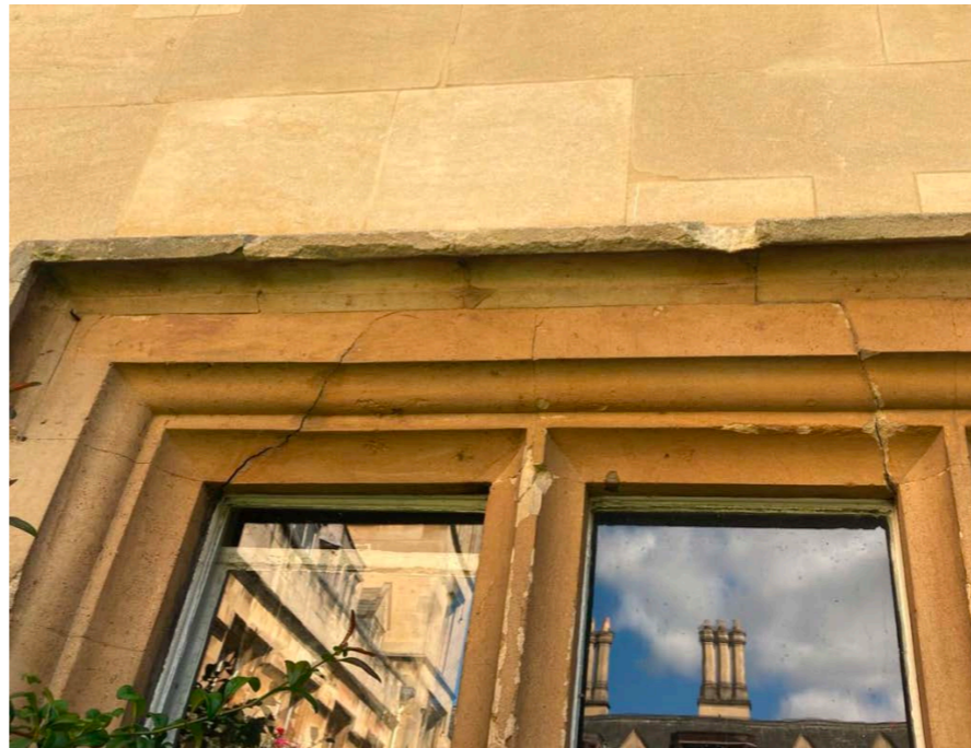
Crack in external stonework
