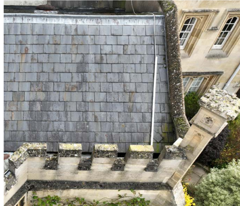
Image from drone survey showing slipped tiles to roof of Broadgates Hall
