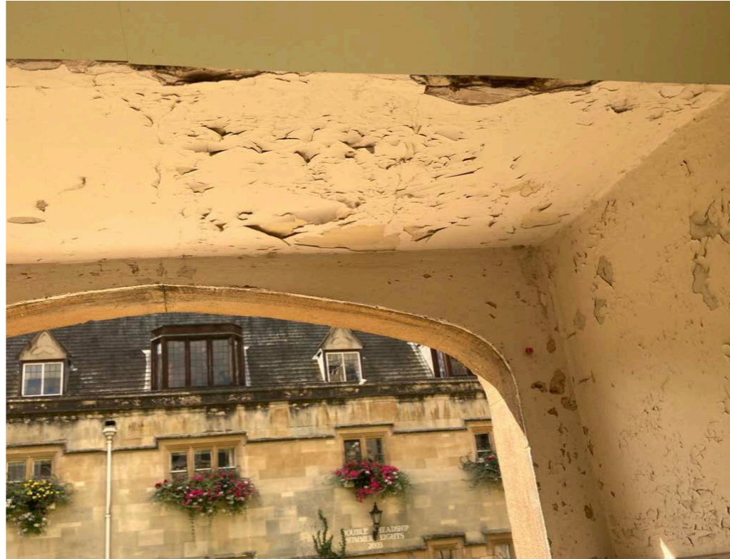
Weathering above door entrance, which has exposed the timber lintel
