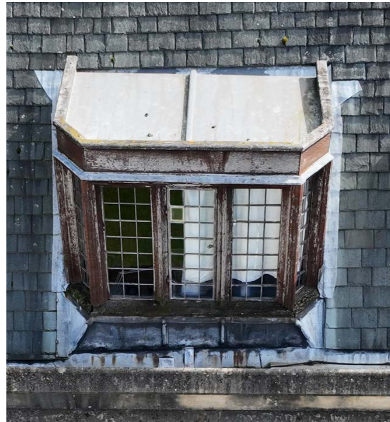
Drone survey image of large timber dormer in Old Quad, showing severe rot to the sill and lower part of the structure and poor protection of parapet detail
