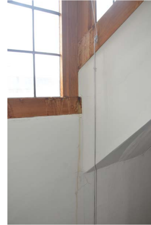
Staining indicating internal water ingress around window panes
