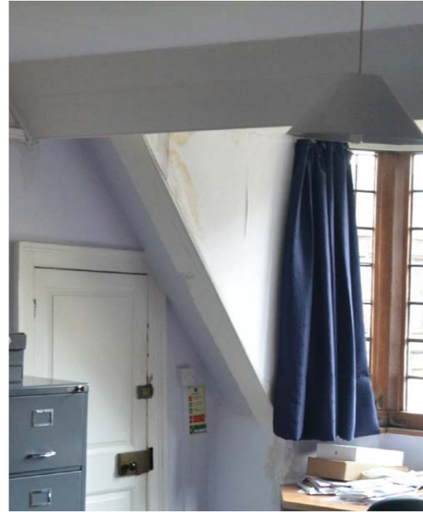
Staining indicating internal water ingress at junctions around dormer windows
