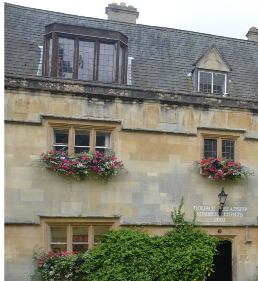
Staining to stone parapet around Old Quad
