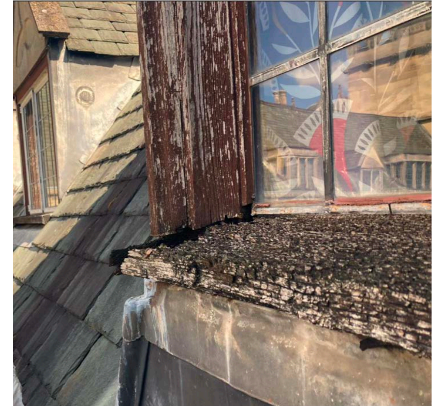
Close up showing severe section loss and deep fissures to sill
