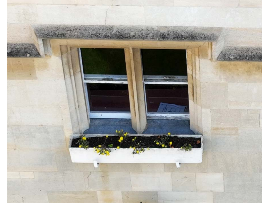
Drone survey image of typical sash window in Old Quad, showing need for redecoration
