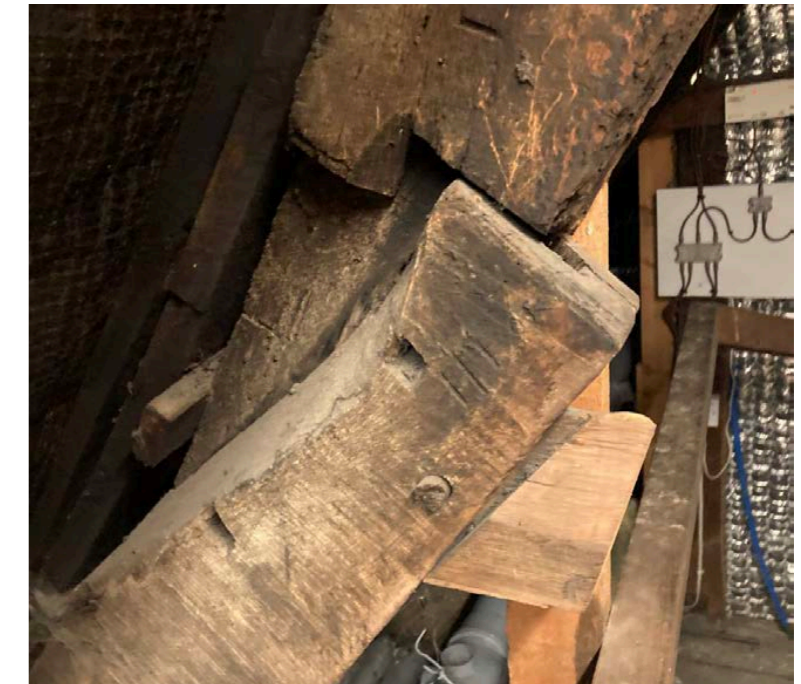
Damaged rafter within loft above Staircase 2
