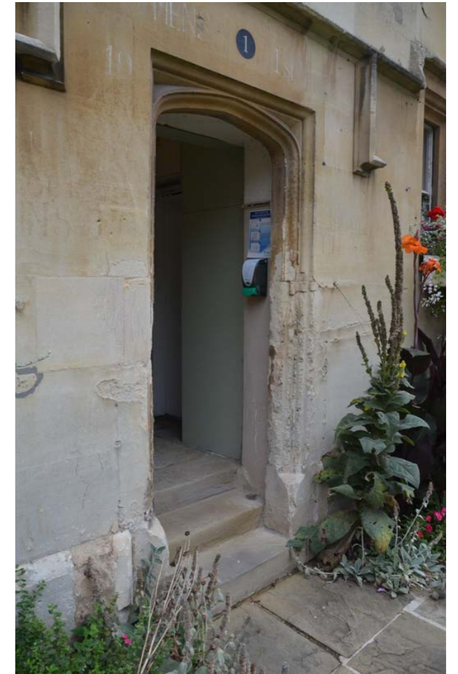
Erosion of stonework around Staircase 1 door
