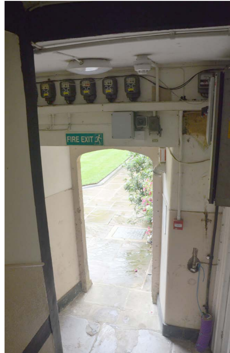
Unsightly electrical installations around Staircase 4 entrance
