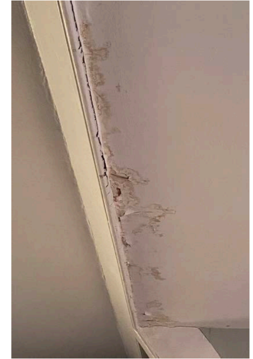
Evidence of water ingress at junction between dormer and roof
