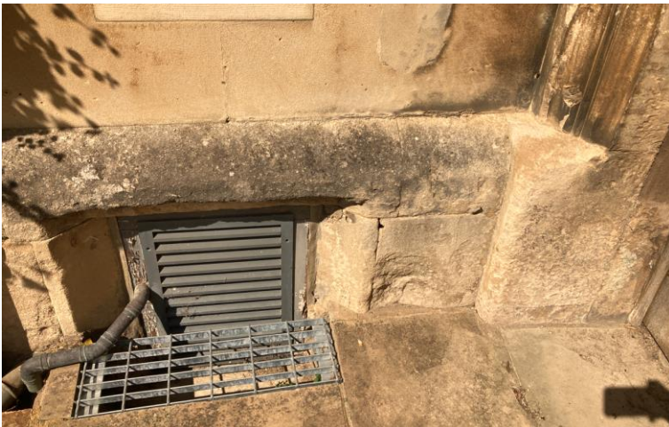
Photograph 27: Erosion to stonework at base of wall
