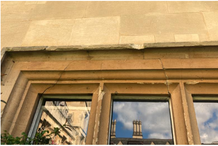
Photograph 26: Crack in lintel above window next to Staircase 3
