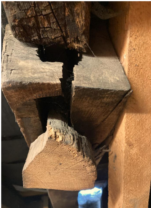
Photograph 13: Split timber rafter
