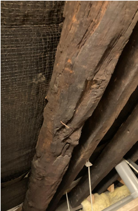
Photograph 14: Timber rafter with section loss
