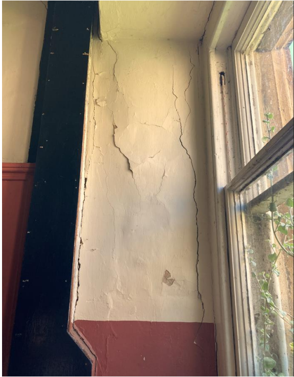
Photograph 4: Cracking in wall on 1st floor landing of Staircase 3
