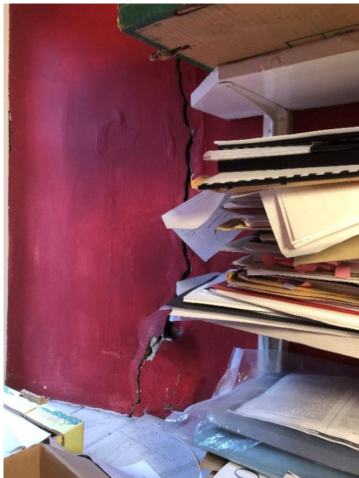
Photograph 16: Crack in cross wall Room 5.9
