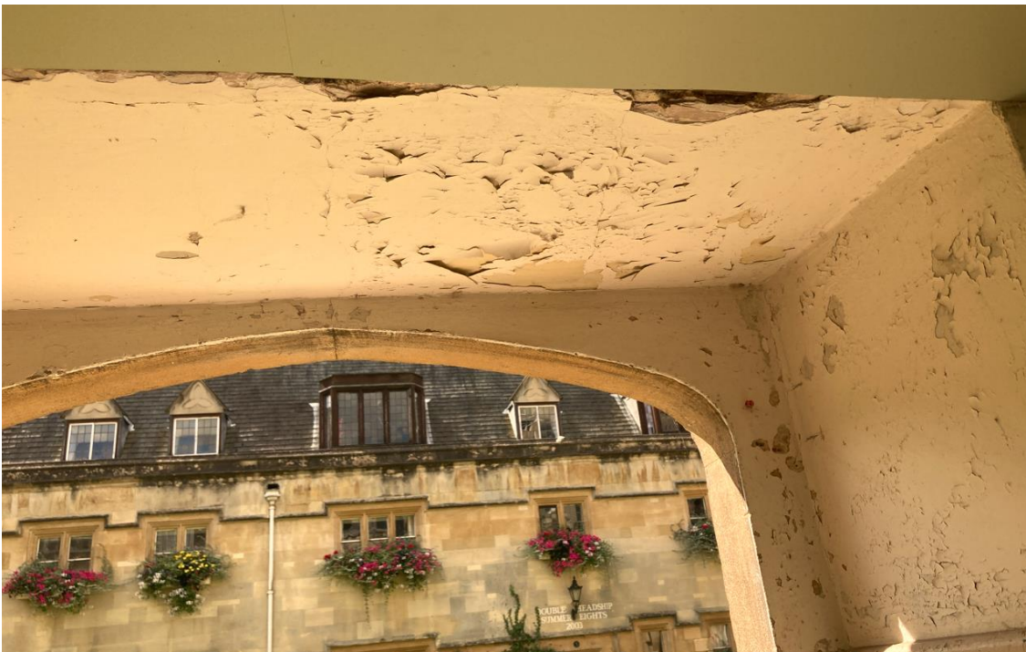
Photograph 3: Ceiling behind entrance arch of Staircase 1 has peeling finishes.
