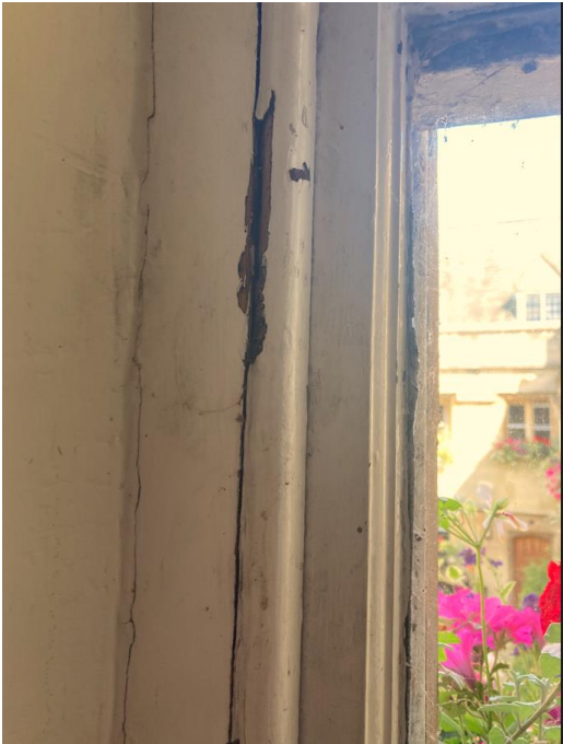
Photograph 8: Section loss in window frame 1st floor Staircase 4
