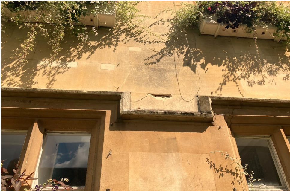
Photograph 22: Section of stone has been lost in wall between Staircase 1 and 2
