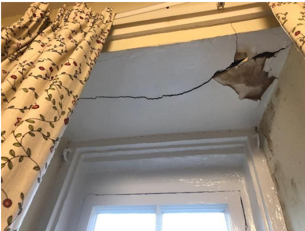
Photograph 20: Cracking to window head in Room 5.1a
