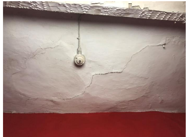
Photograph 21: Cracking to ceiling in Room 5.9
