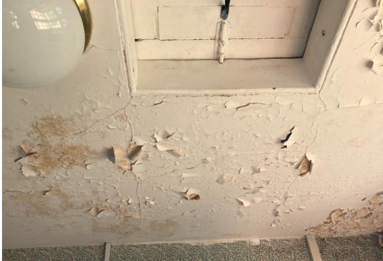
Photograph 9: Paint peeling off ceiling of 2nd floor landing of SCR staircase.
