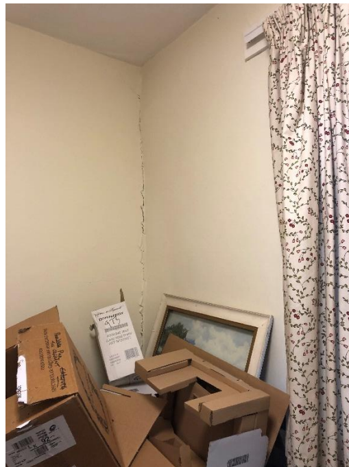
Photograph 17: Crack in cross wall Room 5.1a
