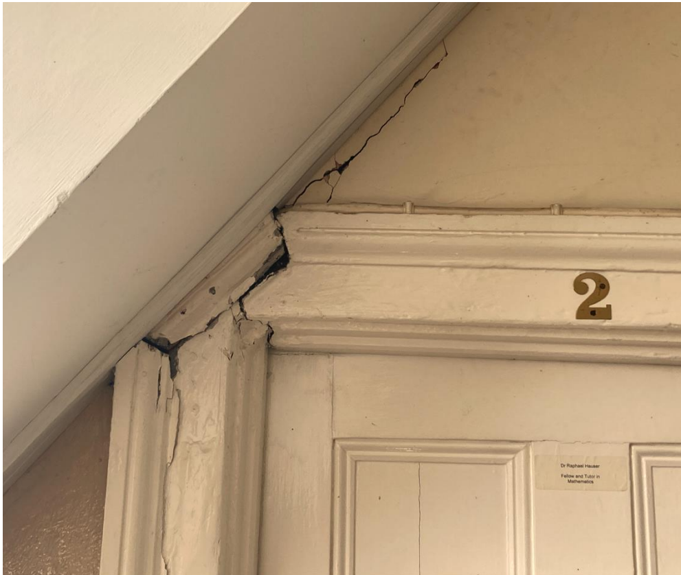
Photograph 1: Cracking above Room 2 on the 2nd floor of Staircase 1
