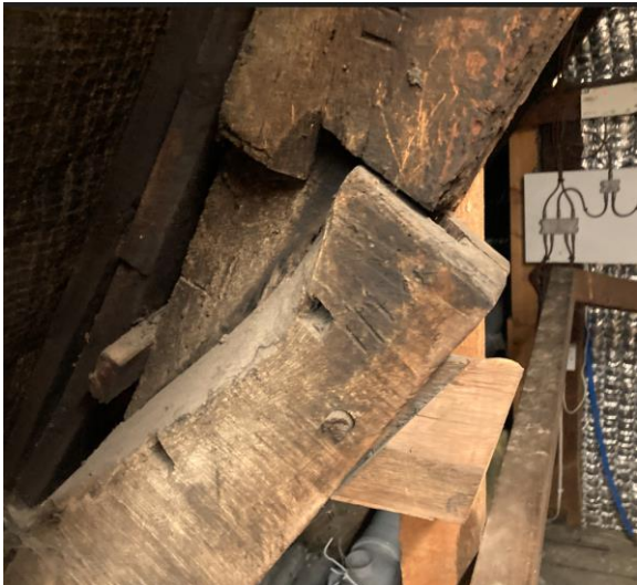
Photograph 11: Timber stump extends 90mm from rafter.
