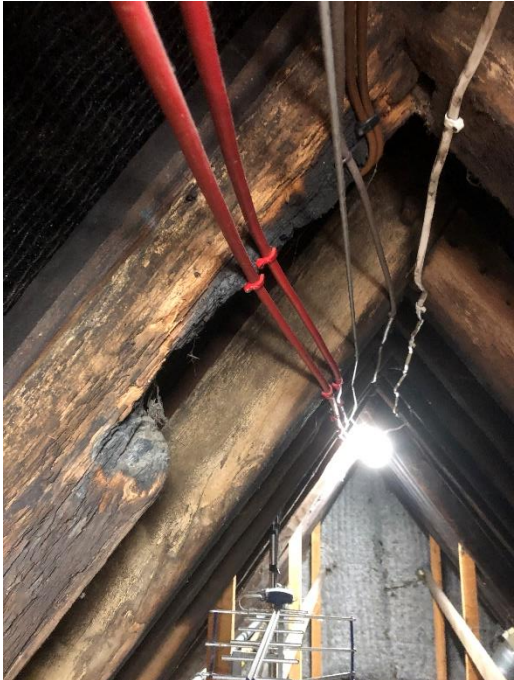
Photograph 15: Fire damage to timber rafter with section loss
