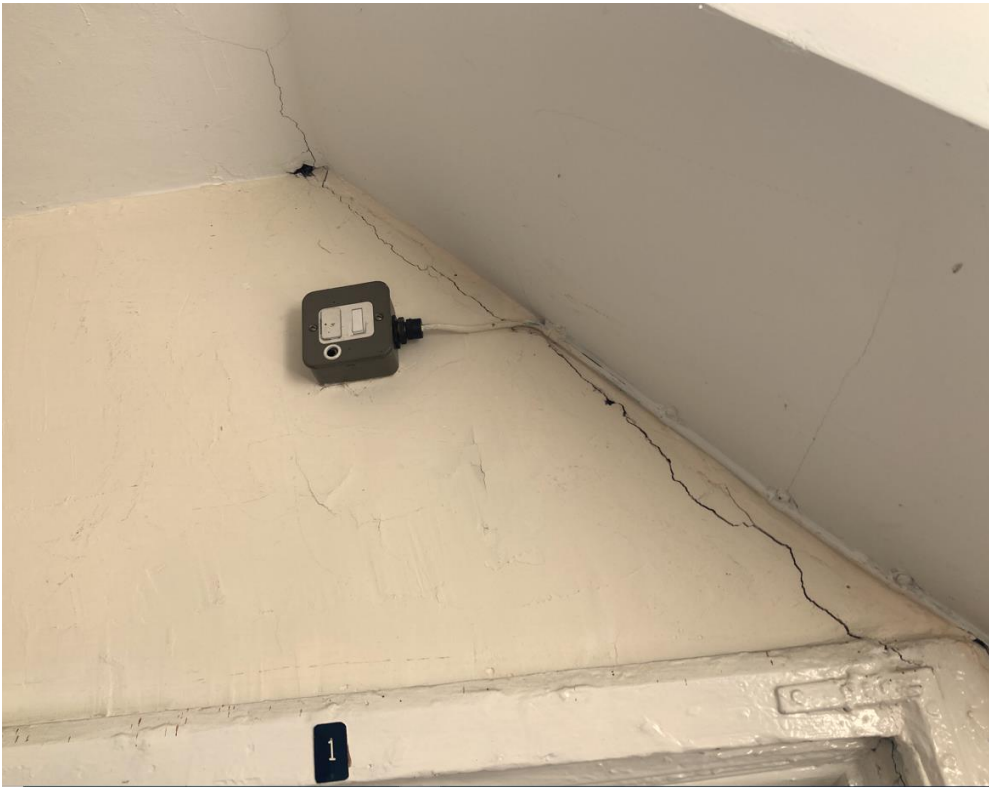
Photograph 2 Crack above door of Room 1
