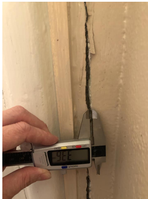
Photograph 7: Measurements of crack 1st floor Staircase 4
