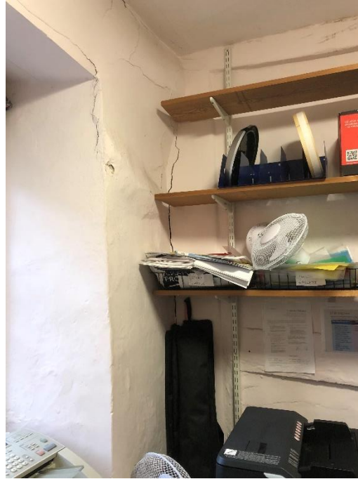
Photograph 19: Further Cracking in Room 5.1a
