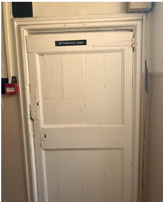
Photograph 6: Crack to right of door on 1st floor Staircase 4
