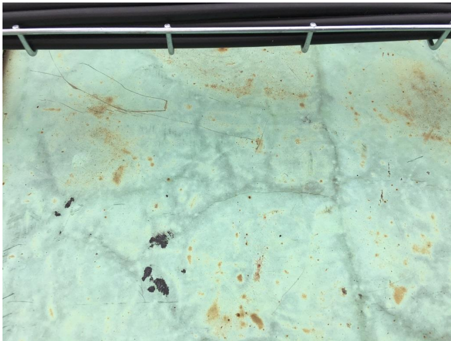
Copper – Crazed surface No 3 – Close up highlighting cracks in the surface of one of the copper bays.
