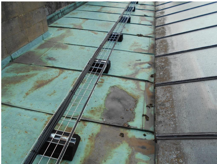
Water ponding on 'flat' surface and patchy patination.
