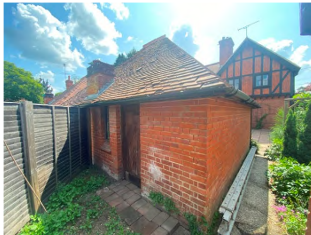
Figure 14: Chimney stack to the rear of the outbuilding in the rear garden of Fielders
