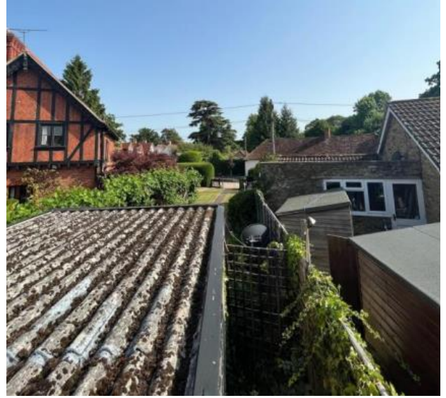
Figure 4: Rear aerial view of perimeter fence between Fielders (left) and Mallow (right)
