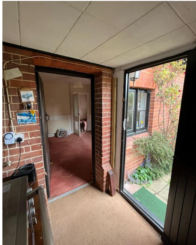
Figure 22: Photograph standing in existing extension facing towards rear of the original building with back door and window
