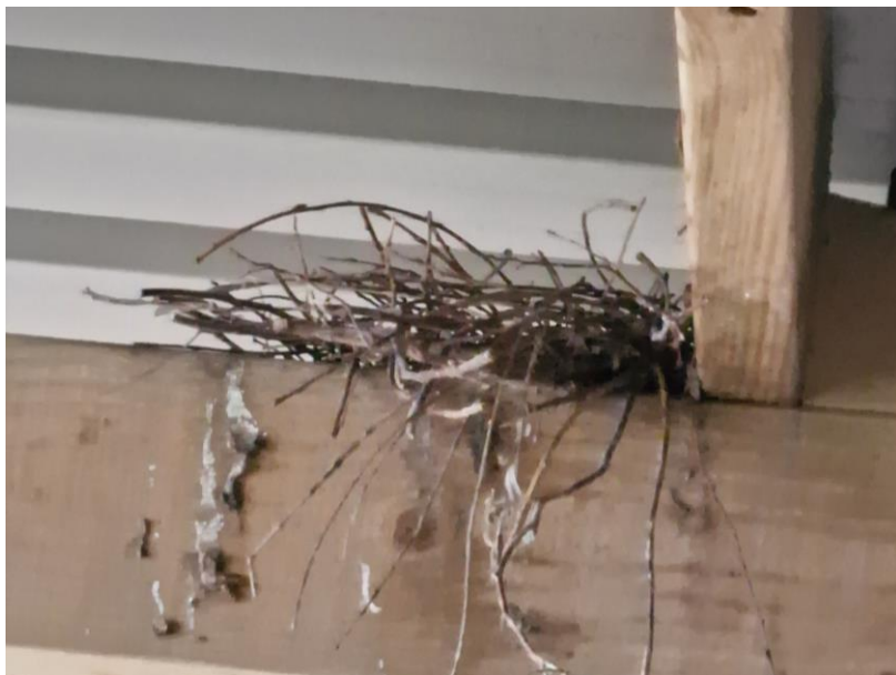
Photo 2: Pigeon nest found on roof truss inside the barn.
