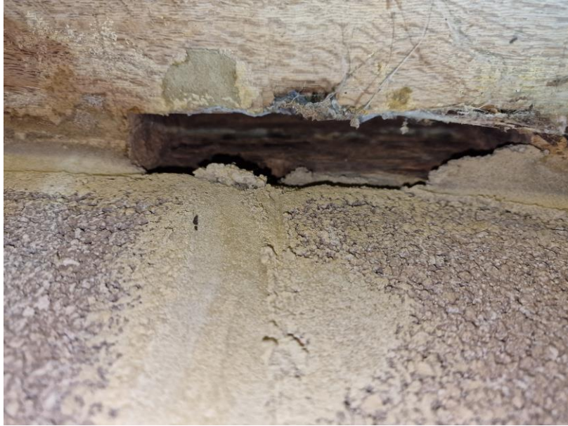
Photo 8: A gap between the brickwork and the roof timber with a bat faeces stuck to the wall.
