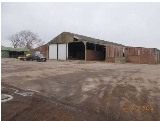
Plate 4: a view of the large barn on the site (Target Note 3). Photograph taken from the south-east. This barn will be demolished and has been assessed to have ‘no’ potential to support roosting bats.
