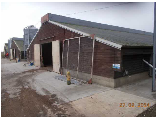
Plate 8: a view of one of the poultry sheds on the site (Target Note 5). These sheds will be demolished and have been assessed to have ‘no’ potential to support roosting bats.
