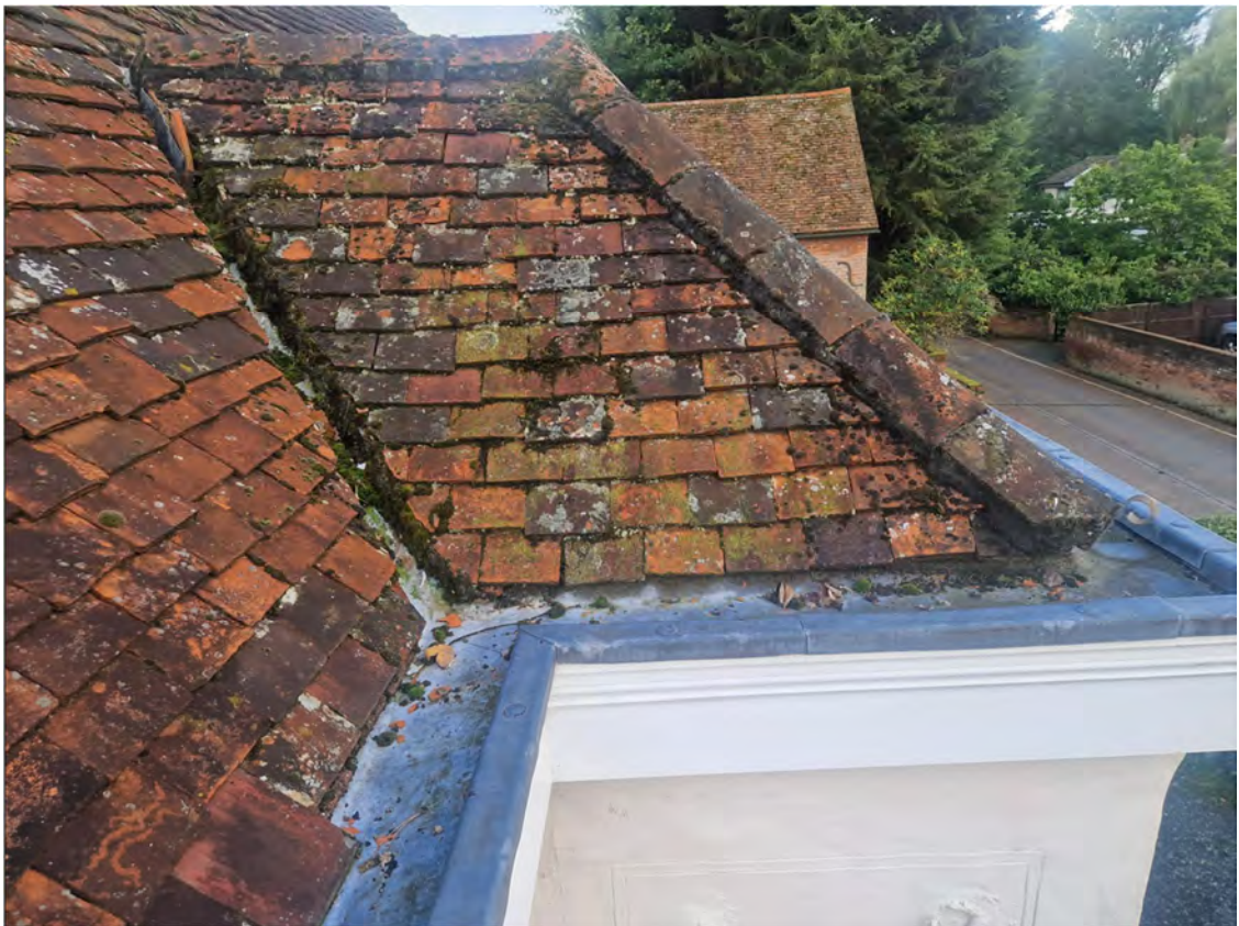
Figure 11. Front roof pitch showing lead box gutter/capping detail and typical tile mix.
