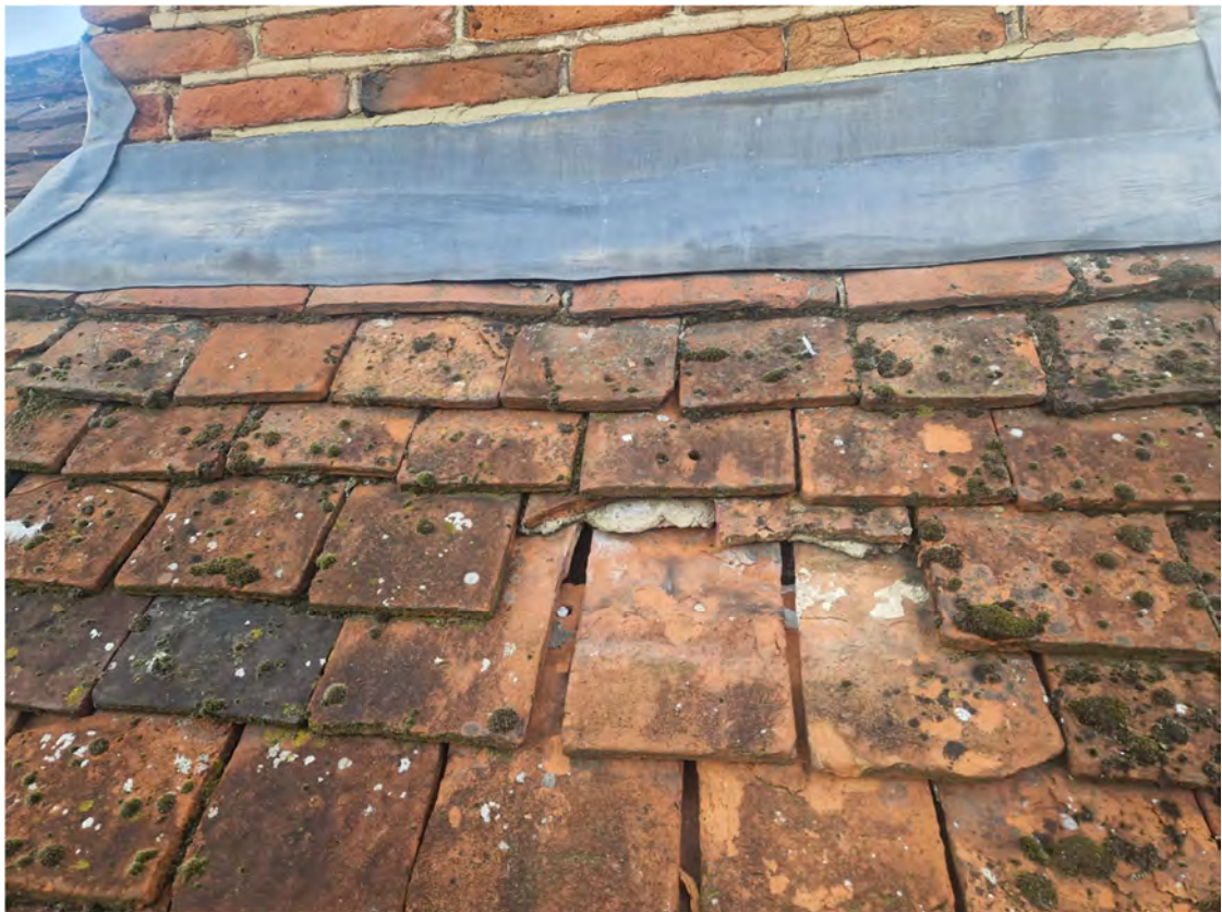
Figures 13a-e. Above and next page- Typical tile deterioration of the main roof, cracked and missing tiles and slippage.
