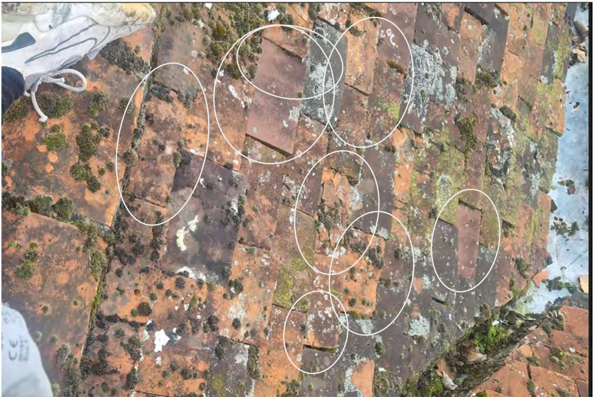
Figure 14. Porch roof with typical unsympathetic machine tile replacement, broken and disintegrated tiles.
