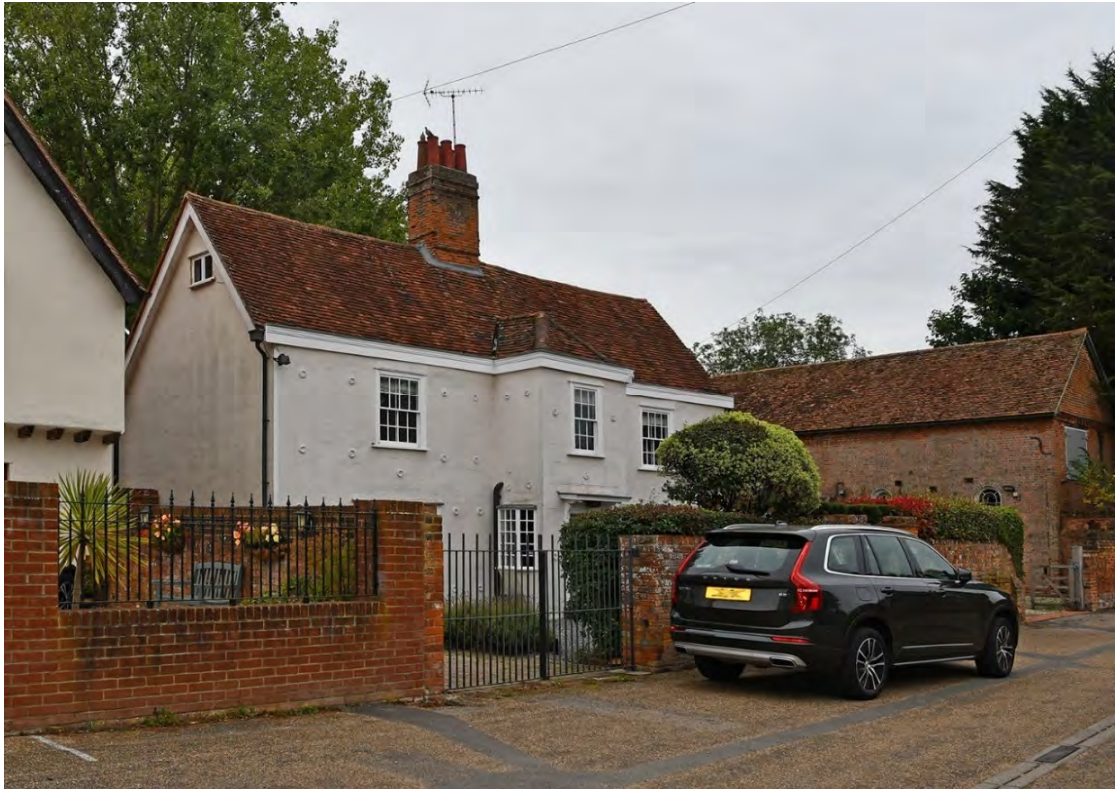
Figure 8. Front from Church Street, for comparison with the above, showing that the eaves box gutter detail is not historic.
