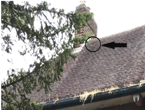
Missing roof tiles on east aspect of roof (circled and arrowed)
