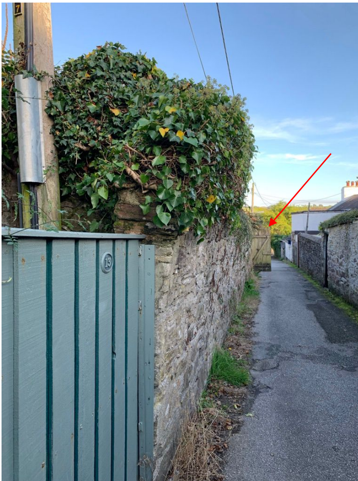
Arrow indicated existing gateway onto the site. Note the outward lean of the rubblestone wall
