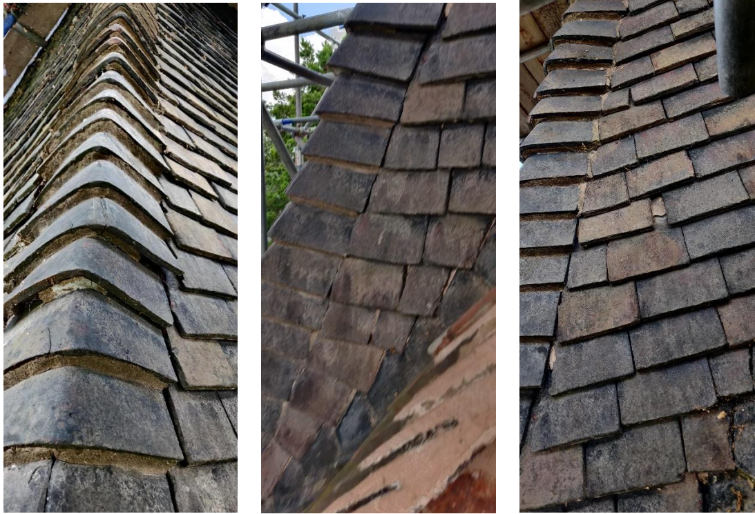
Fig 3. Photographs showing existing bonnet hip detail to lower section of Bell Tower.
