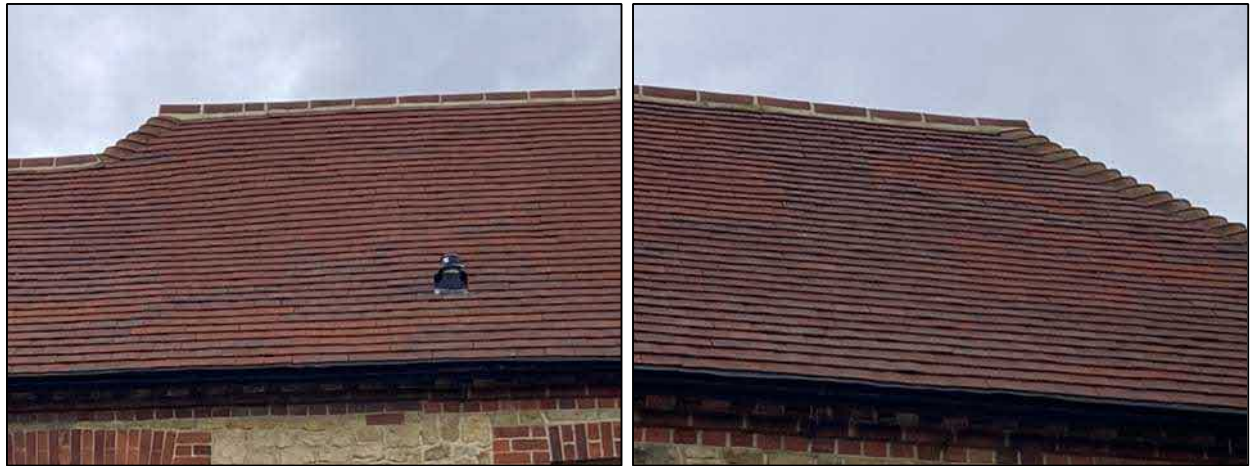
Photograph 3a (left) & 3b (right). Views of the eastern pitch of the roof, showing lifted tiles with suitable features for roosting bats.
