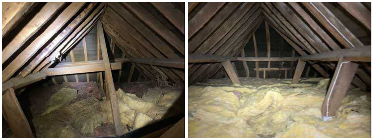
Photograph 5a (left) & 5b (right). Views of the main void space, where scattered bat droppings were identified.
