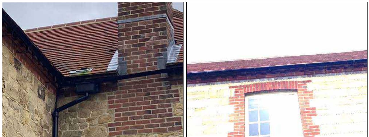
Photograph 4a (left) & 4b (right). Left – View of the northern elevation of the building, showing gaps around hips and the chimney. Right – View of the eastern eaves with possible access gaps into the loft voids.
