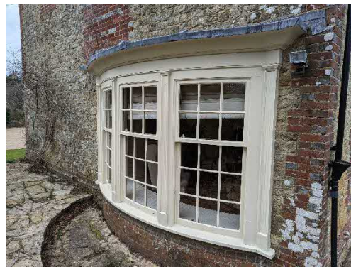
Figure 8 – Existing lead flat bow window to have a new lead pitched and scalloped roof.
