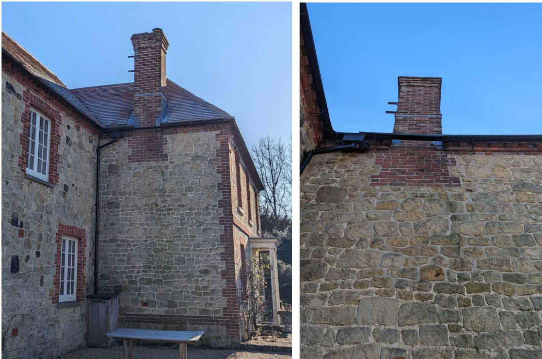
Figure 9 – Existing north facing chimney and detail photo of poor pointing in suspected cement mortar
