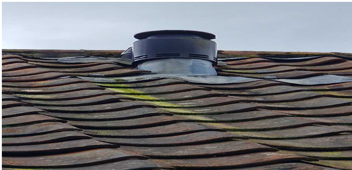
Picture 2: Showing the gaps under the tiles on the front elevation of building 1
