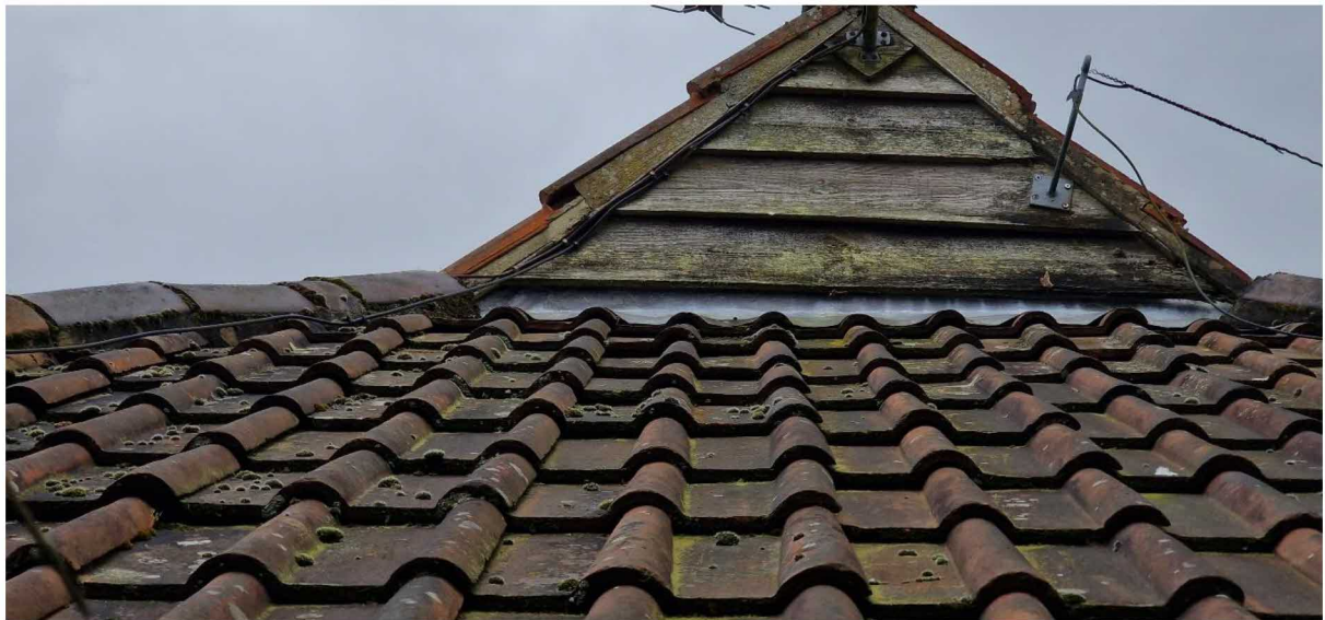
Picture 6: showing the weather boarding and the missing cement on the tile verge (building 2)
