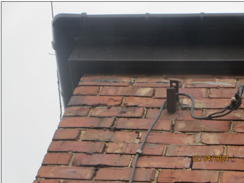
Figure 11. Gaps are present behind fascia boards.
