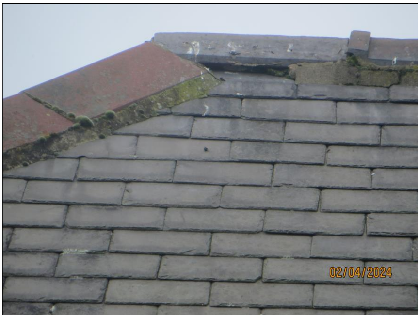
Figure 12. Gap present below ridge tile.
