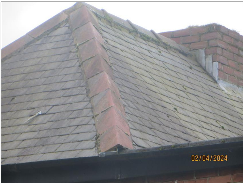
Figure 16. Possible gap at bottom of hip tile on north eastern corner.
