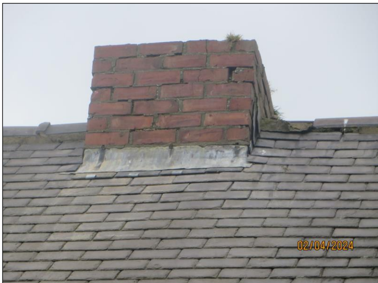
Figure 13. Pointing absent around sections of the chimney.
