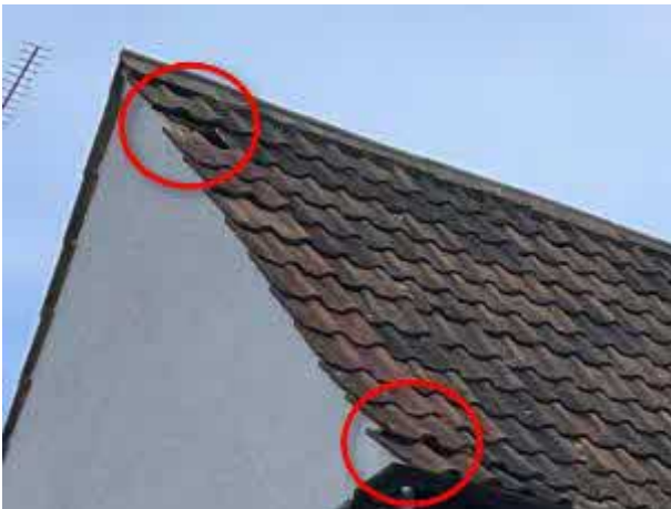
Plate 13: Missing and slipped roof tiles on south Pitch of structure 1.
