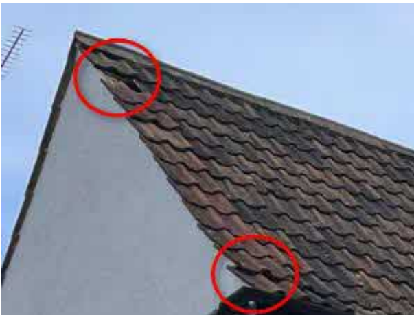
Plate 13: Missing and slipped roof tiles on south Pitch of structure 1.
