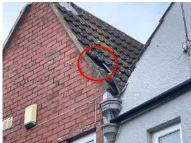
Plate 14: Missing roof tile on south pitch of structure 2
