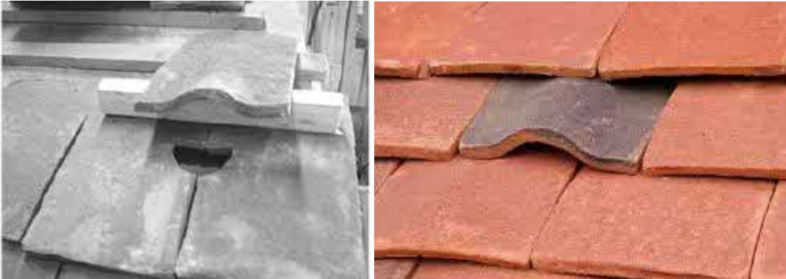
Figure A6.1. Roof slope crevice roost bat access tile suitable for areas of clay tiling. Bespoke lead access tiles can also be used.
