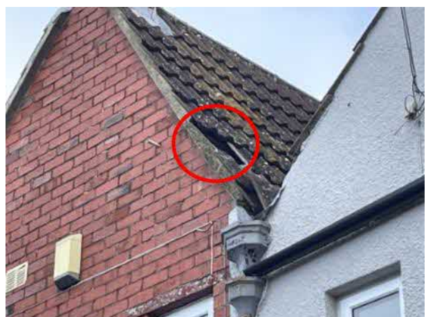
Plate 8: Missing roof tile on south pitch of structure 2
