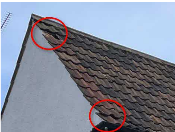
Plate 7: Missing and slipped roof tiles on south Pitch of structure 1.
