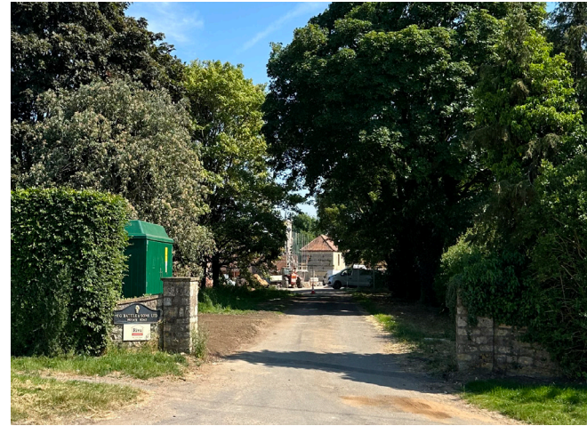
View looking south towards the existing drive adjacent to the development site, where the scheme for 16 dwellings is under construction.
