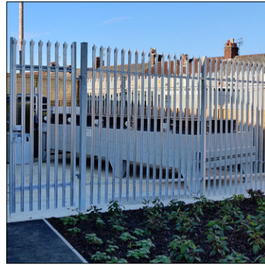
3 Palisade fencing, 2.5m high to external refrigeration plant cage and rear of store. Finish - galvanised
