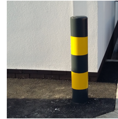
4 Galvanised steel heavy duty bollard with concrete infill, painted black and yellow
