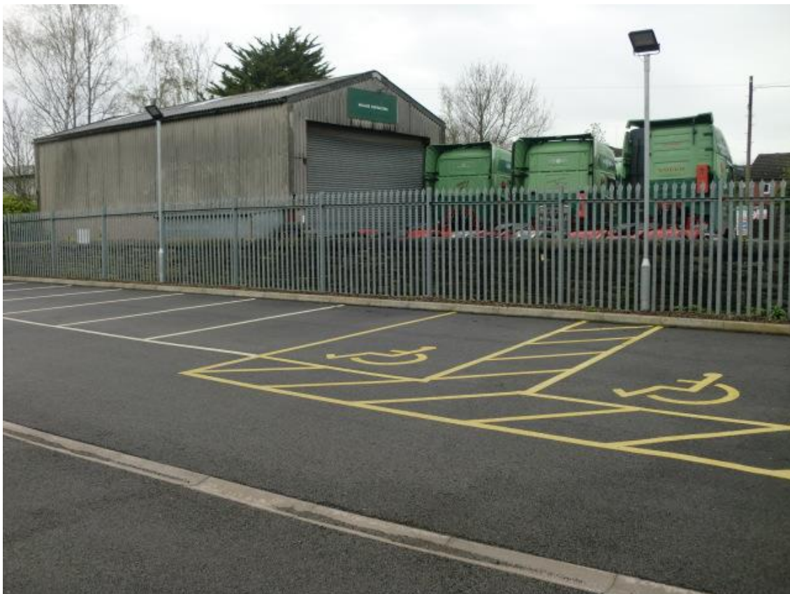
Figure 1: Image of light columns in car park
