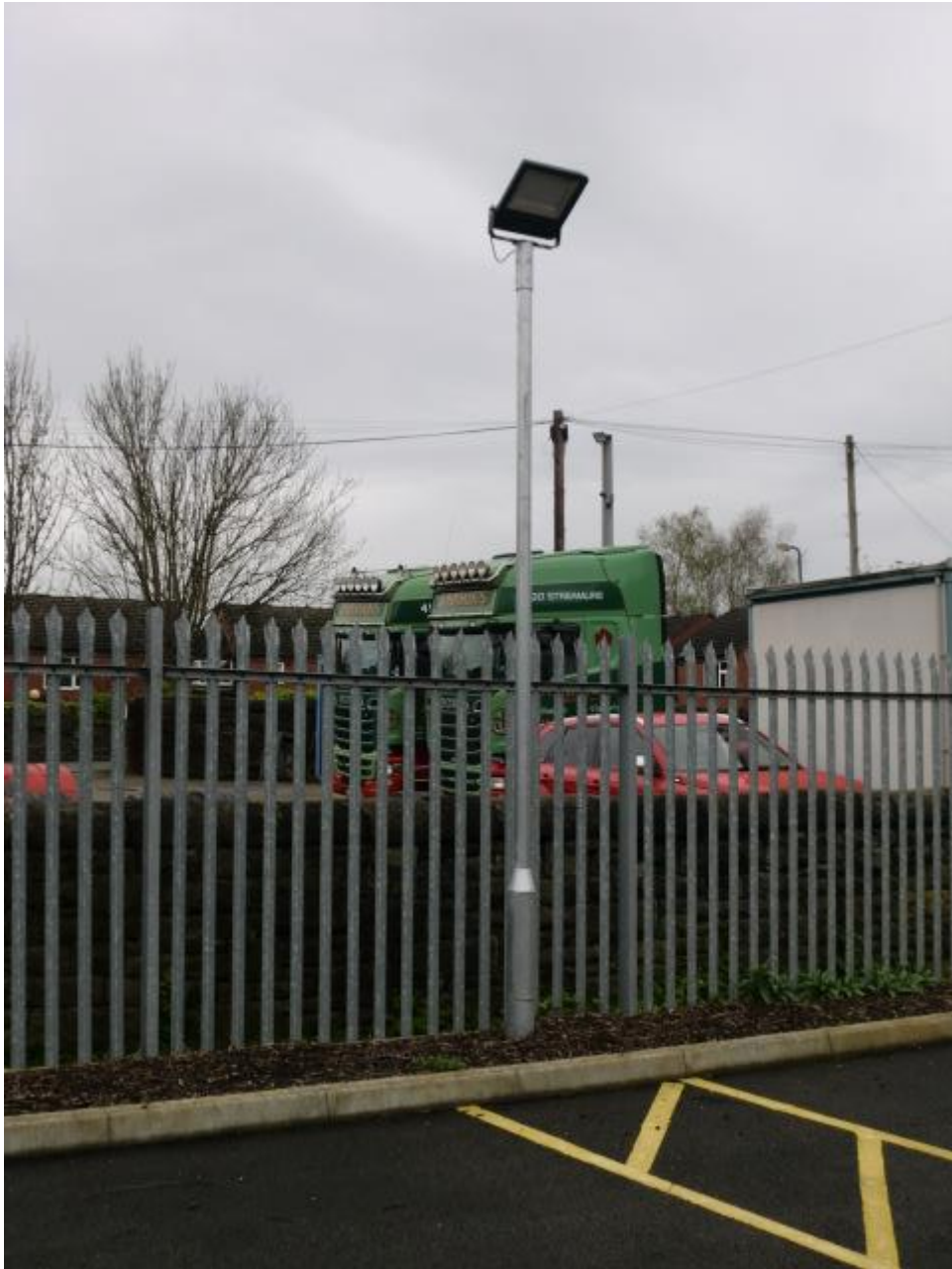
Figure 2: Light column in car park
