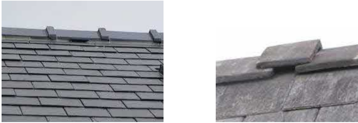
Figure 1: Gap in mortar (left); raised ridge tile (right)
