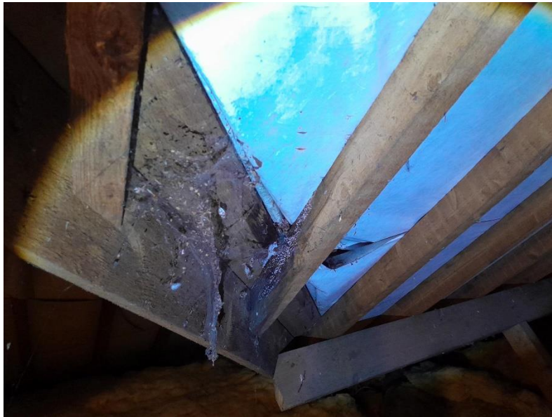
Photo 8. Gap in roof lining where light penetration occurred – Void B.
