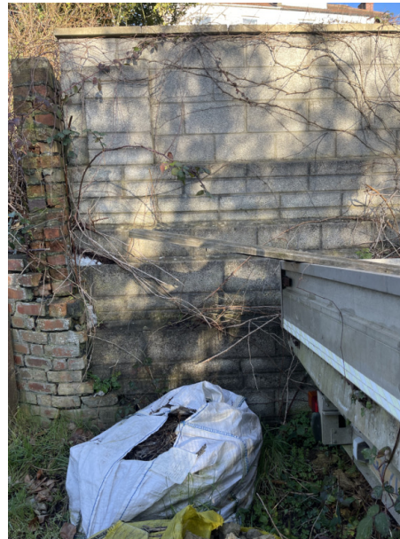
Section of existing garden retaining wall, part of which would be strengthened by walls of proposed new garage/annex
