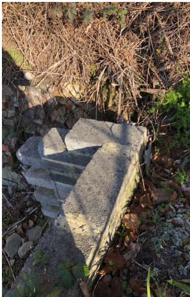
Corner of the concrete blockwork wall built by the owner to provide additional support to footpath steps
