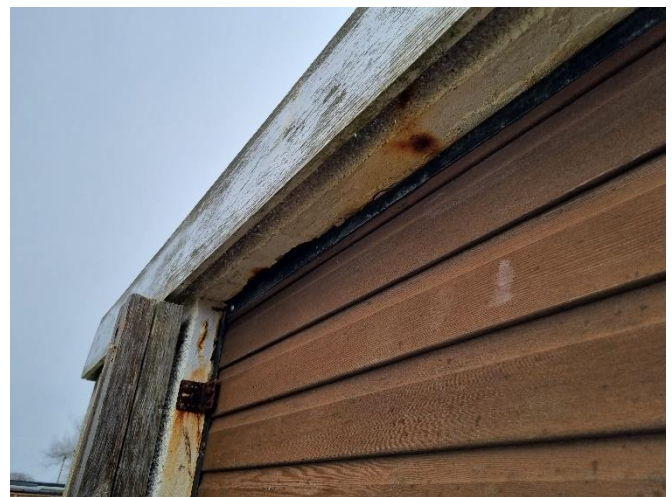
Photo 2: Single garage door gap
