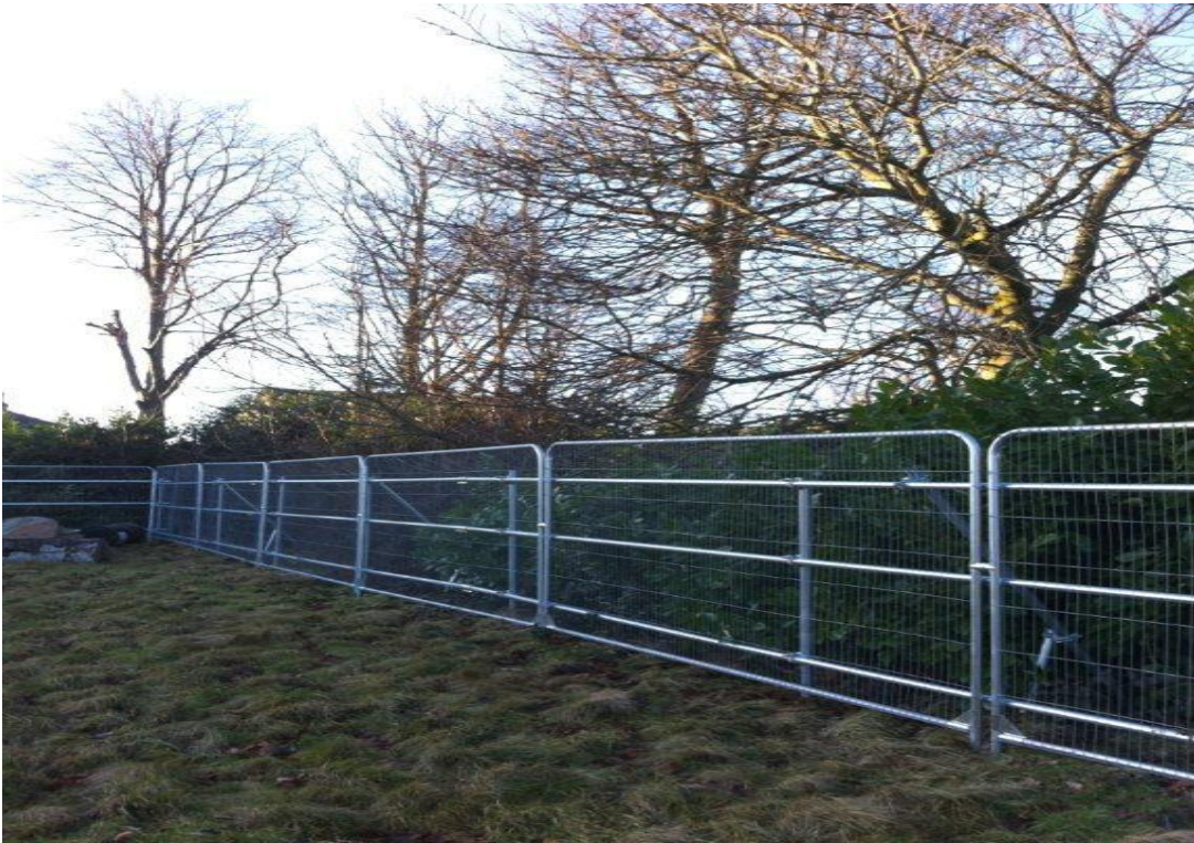
Figure 1 Photograph 1. Example of BS5837:2012 Tree Protective Fencing
