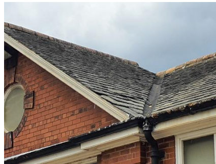
Figure 7 Uneven tiles at gable.
