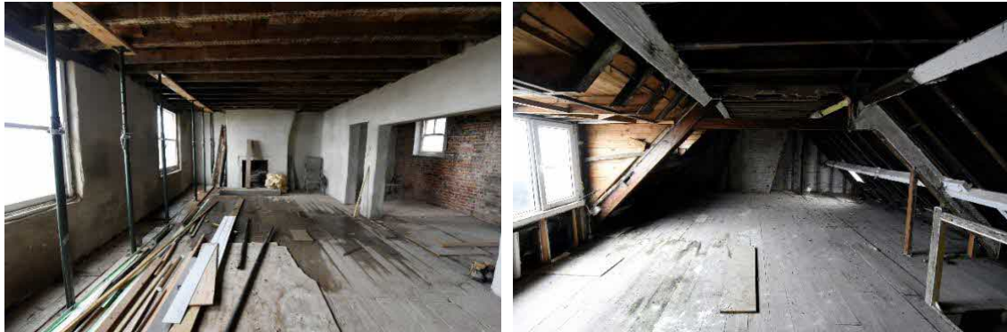
Figure 12, All internal walls, doors, ceilings and other fixtures have been stripped out of the property on all floors.
