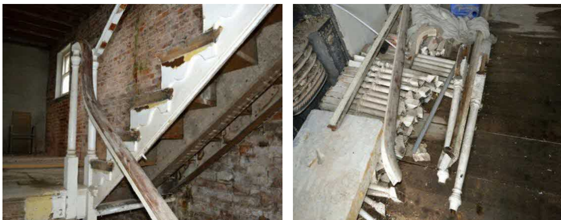
Figure 10, Late 18th to early 19th century ramped staircase, which has been dismantled during recent renovation works.
