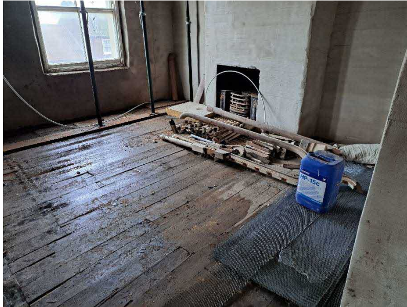
Typical internal condition showing first floor western gable and front elevation with water ingress, structural propping and partially dismantled stair components.
