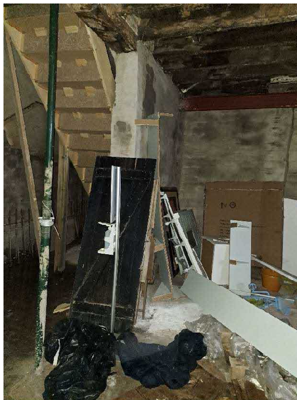
Typical internal condition showing the ground floor stairwell in the North East corner with temporary flight to the first floor and most of the period features now removed by previous owner(s).
