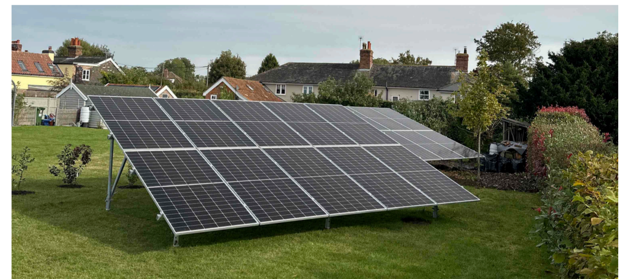
Example picture of same panels recently installed elsewhere by Electricians
