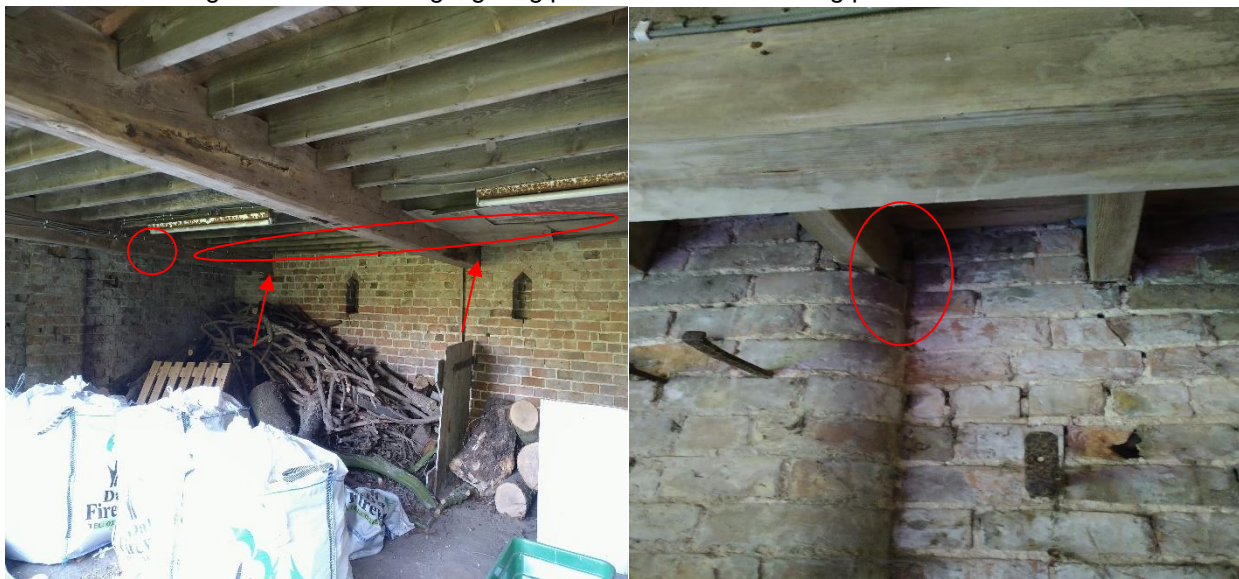
Plate 4.5 – (L) – Facing SW, Room 3 highlighting potential roosting points (R) – Bat droppings highlighted in the joist puttock hole on the south elevation.
