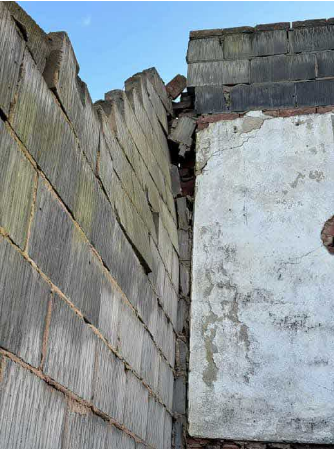
RIGHT HAND SIDE GABLE – STRUCTURAL DEFECTS FROM THE INSIDE
