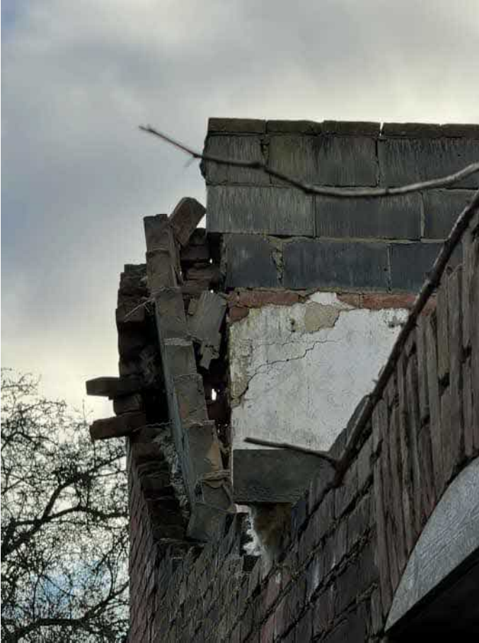
RIGHT HAND SIDE GABLE – STRUCTURAL DEFECTS
