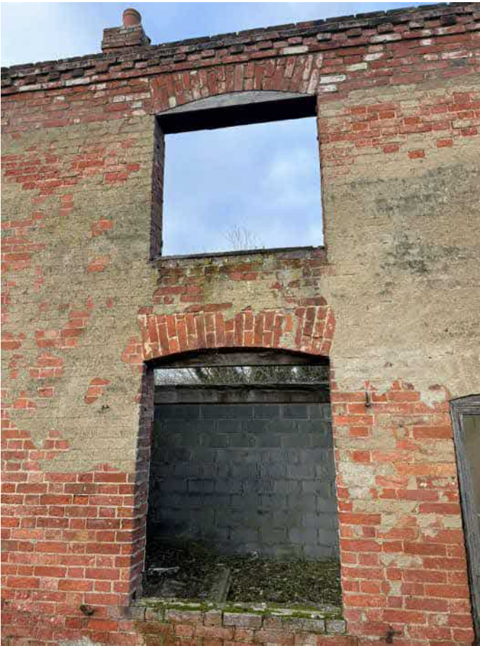
FRONT ELEVATION - STEPPED FRACTURES ABOVE GROUND FLOOR WINDOW
