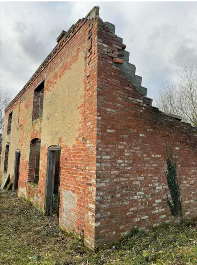
FRONT / RIGHT HAND SIDE ELEVATION – STRUCTURAL DEFECTS TO BUILDING CORNER
