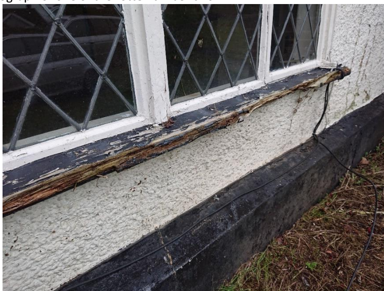
Fig 3. Photograph of one of the rotten timber cills
