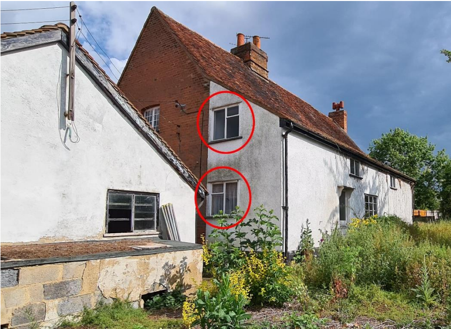
Fig 5. Side elevation (north) mid-20 th century metal framed windows to be replaced.
