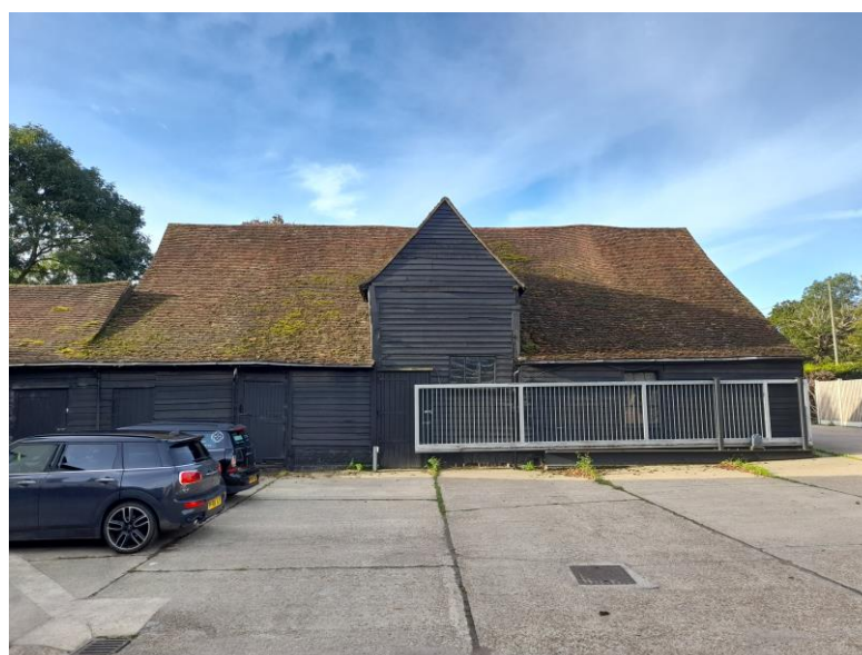
Image 12 Front elevation of Grade II listed Barn to West of Pursley Farmhouse
