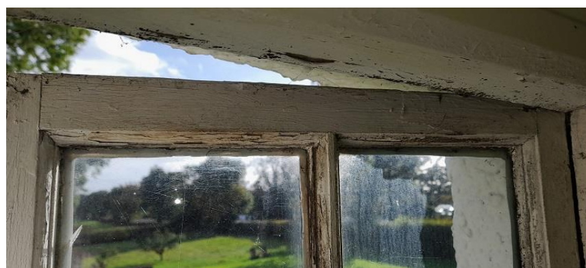
Image 7 Swollen frame has made window very difficult to open, with subsequent hazardous black mould around entire frame & glazing bars
