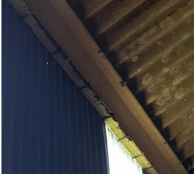
Above: Spalling to underside of gutter / eaves beam
