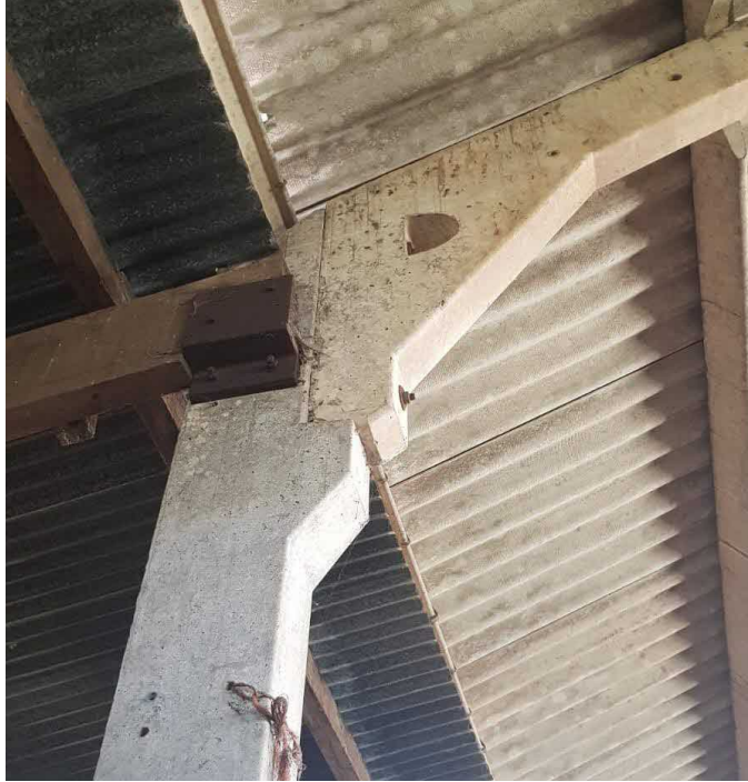
Above: Typical moment connection at the eaves of the pre cast concrete frames
