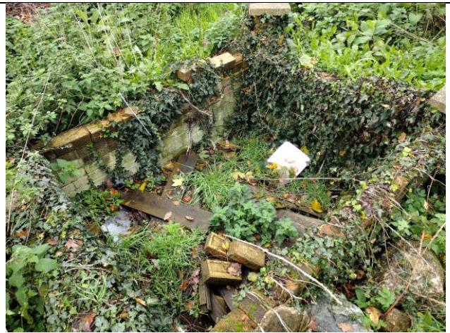
Photo 10: Low brick walls with loose bricks within the garden area.
