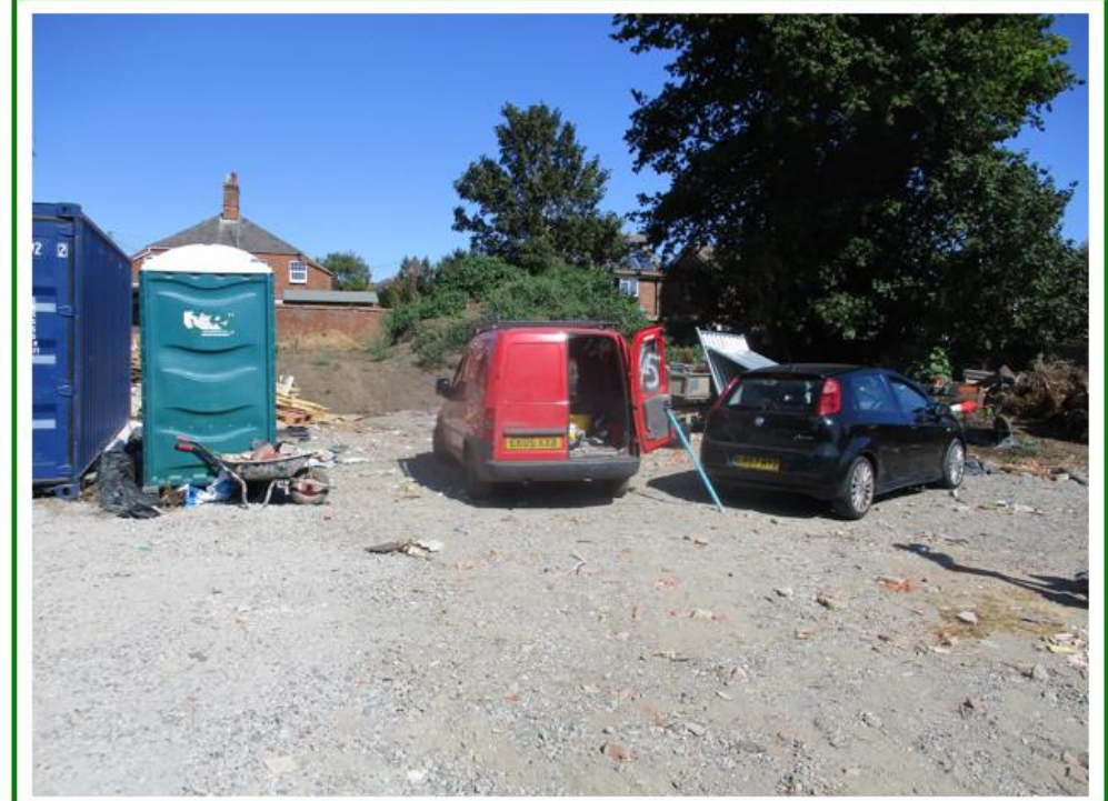
Photo No.2: Facing north from the southern site boundary showing parking and staging area for site works
