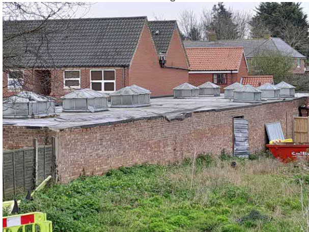
Derelict commercial building
