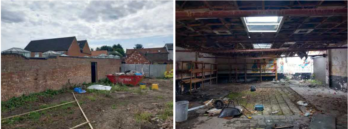
Plate 27: Image of the exterior and interior of the flat roofed commercial building
