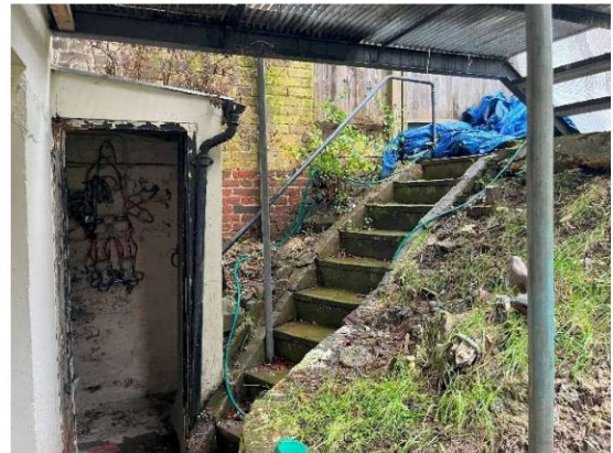
Outhouse W/C and stone/concrete steps
