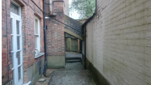
Image 6. Old Boiler Room walkway with view of bridging flue (to be demolished).
