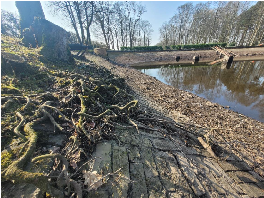
Photograph 12 – Extensive root over-growth and damage along dam structure
