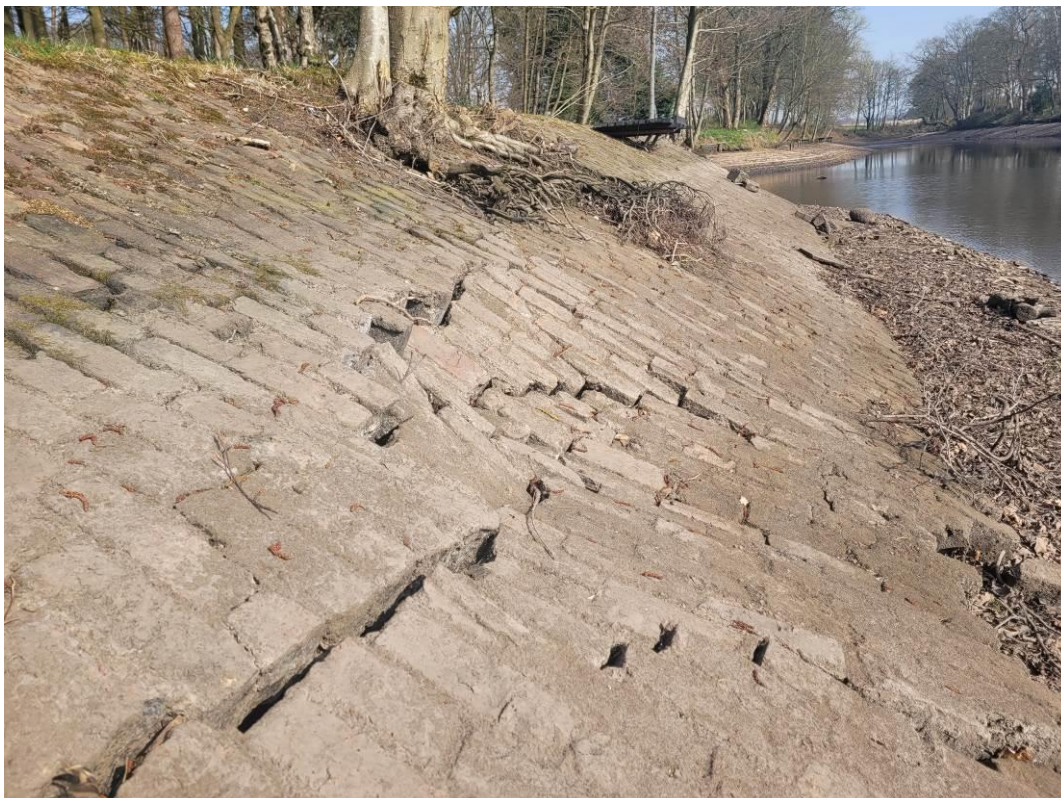
Photograph 11 – Cracking to dam structure caused as a result of extensive root damage and lack of maintenance.
