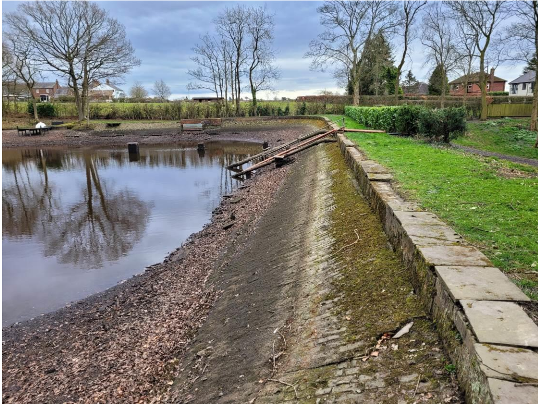
Photograph 10 – Extent of brick-built dam structure (water level temporarily reduced during routine maintenance)
