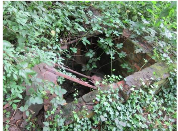
20 – Drawoff siphon valve chamber overgrown
