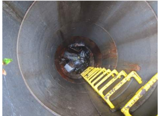
25 – MH5 new manhole immediately upstream of road crossing, flow enters from upper left
