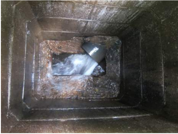
22 – MH2 overflow A flowing and entering existing pipe from overflow B
