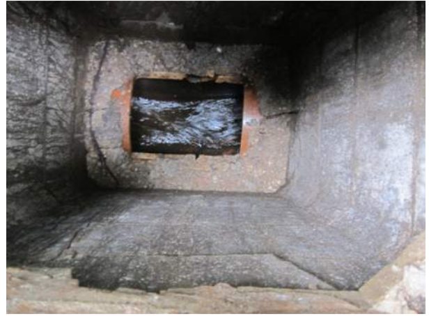
23 – MH3 within car park
