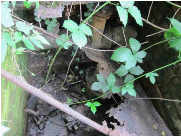
21 – Drawoff siphon chamber internals
