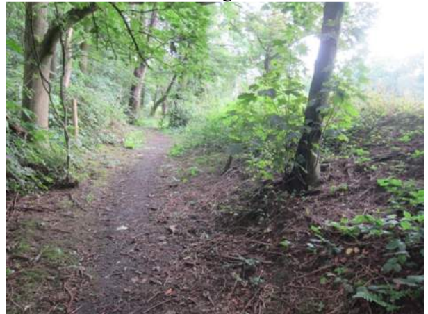
10 – Embankment downstream face at right return, the right abutment is in the distance
