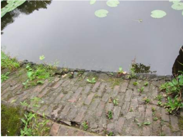
17 – Crack in brick wave protection downstream of overflow B, which is to the immediate right.
