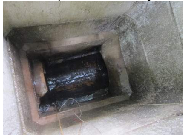
22 – MH1 no flow from overflow B
