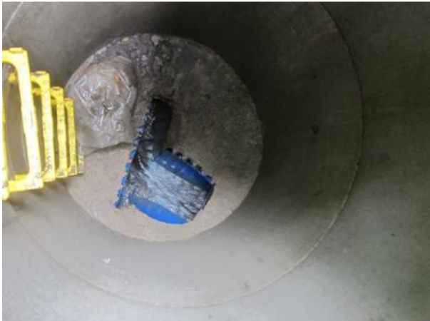
24 – MH4 new manhole, mitred bend liable to catch debris but currently appears clear, flow enters from right
