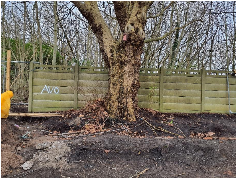
Figure 2 T2 Evidence of root severance and excavation within RPA.
