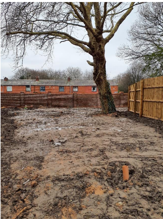
Figure 4 T9 evidence of compaction from tracked machinery.
