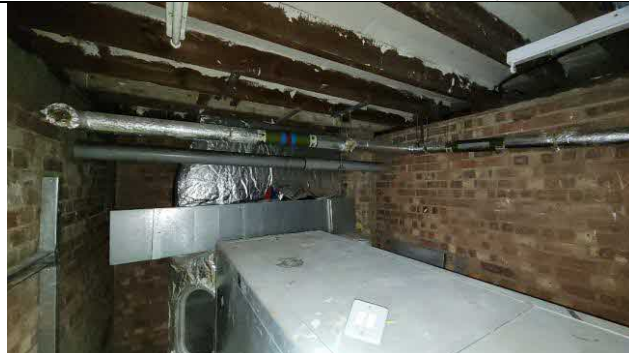
Photo 23: Non-operational boiler room on the fourth floor.
