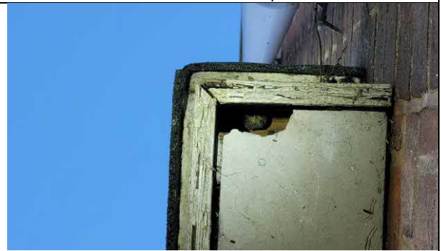
Photo 16: A gap on the fascia board, creating a PRF on the one-storey section on the southern aspect of the Building 1.
