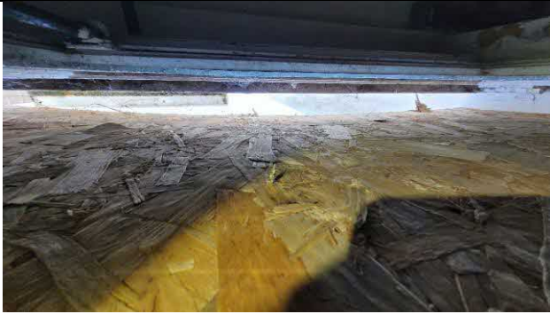
Photo 25: Gap created with unsealed chipboard
