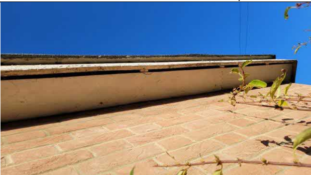
Photo 15: PRFs within the soffit box on the one-storey section on the southern aspect of the Building 1.
