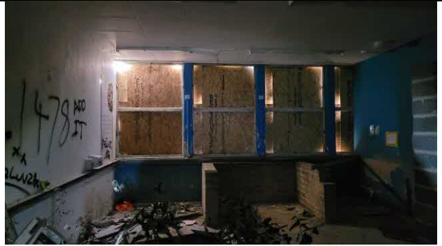
Photo 18: Gaps within the chipboard on the southern aspect of Building 1.
