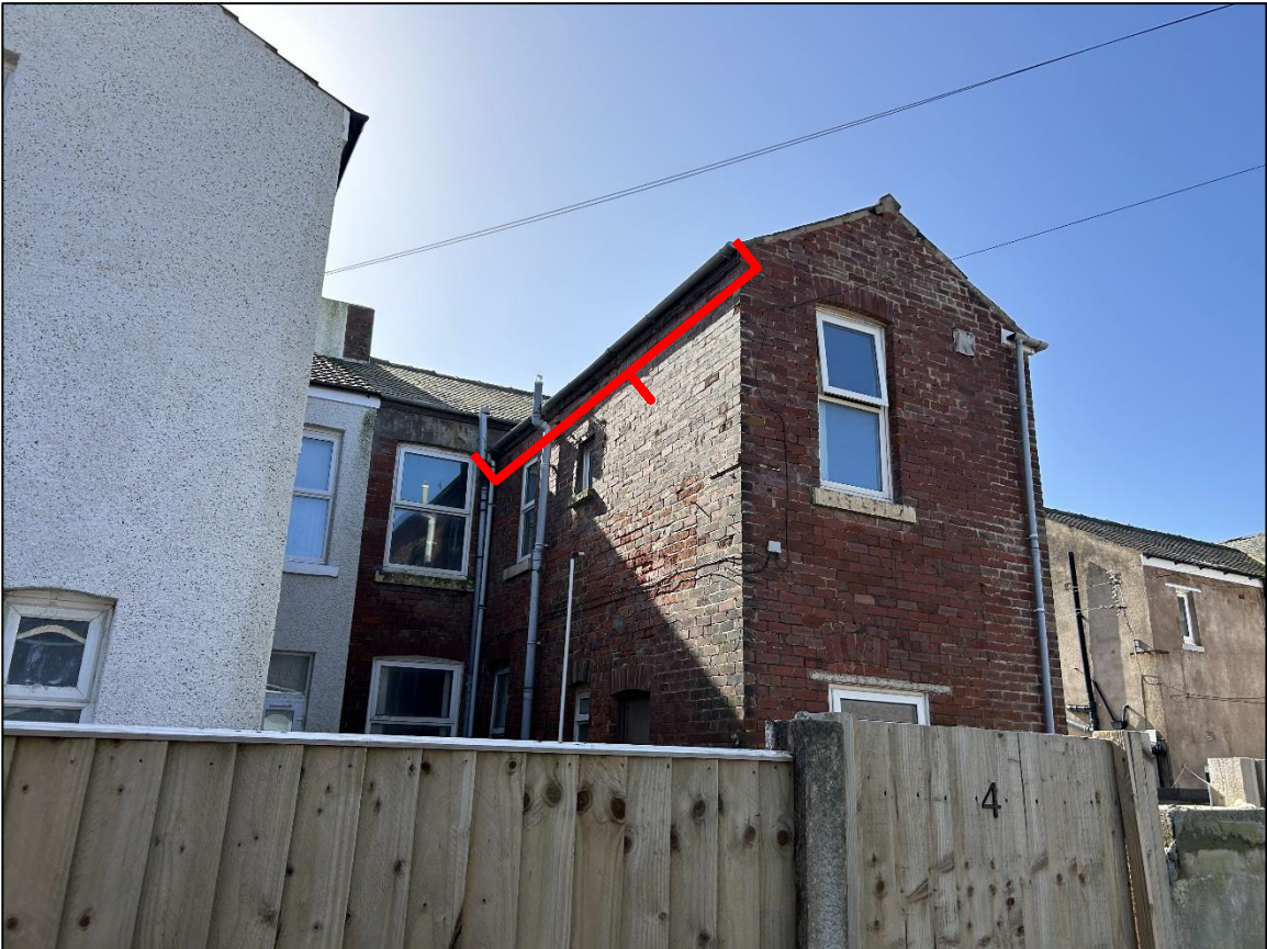
Plate 6 – Eastern facing aspect, with gaps beneath timber fascia
