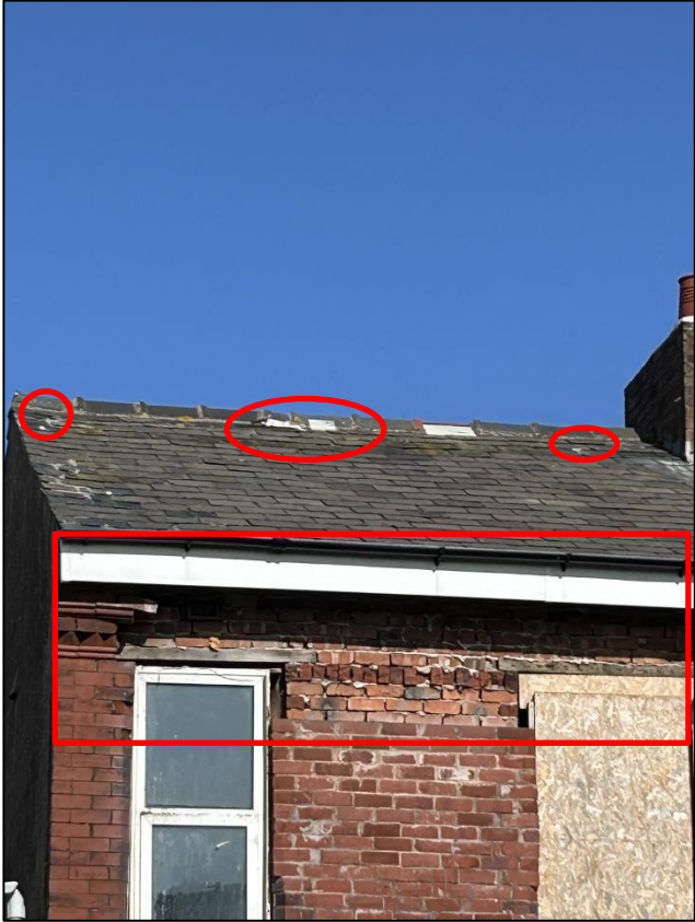
Plate 2 – PRFs on southern elevation, circled
