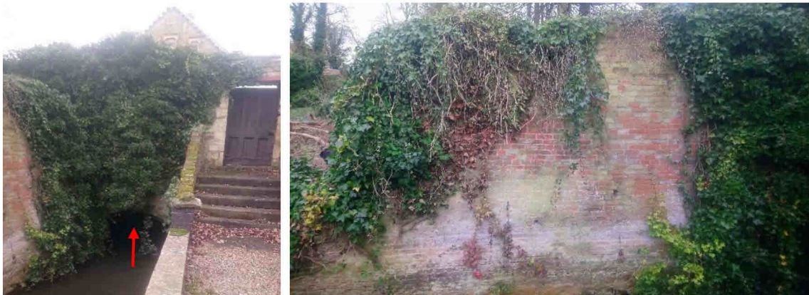
Culvert under Abingdon Rd reported used by roosting bats & adjoining walls with dense ivy/holes
