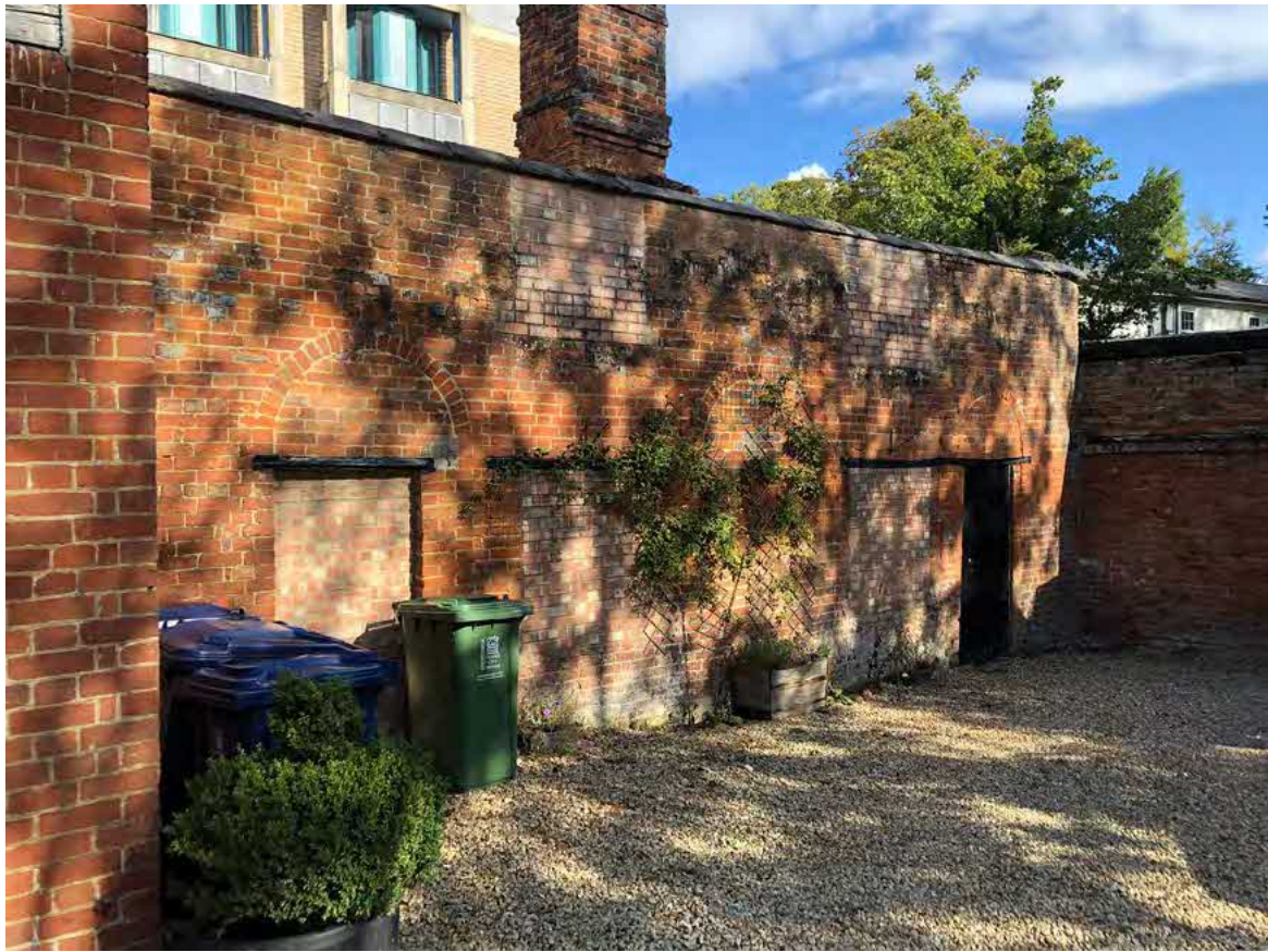
Plate 5: Derelict building at the end of the old stable building
