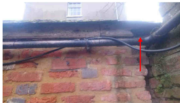
B3, hole in barge point/possible entry point SW cnr
