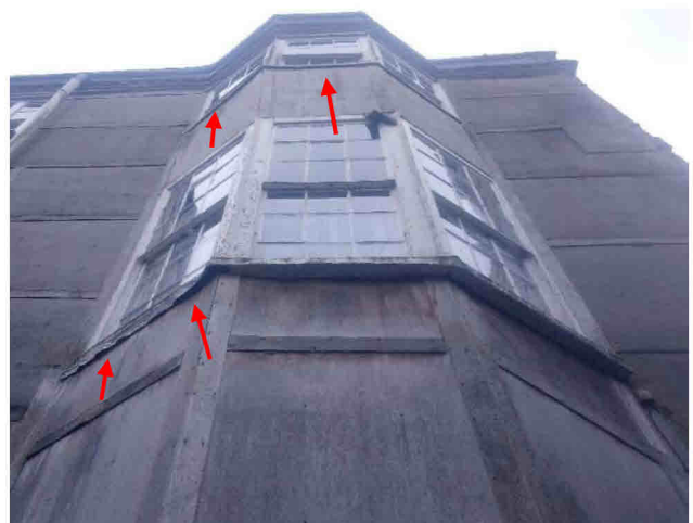
B5, gaps under lead flashing beneath windows
