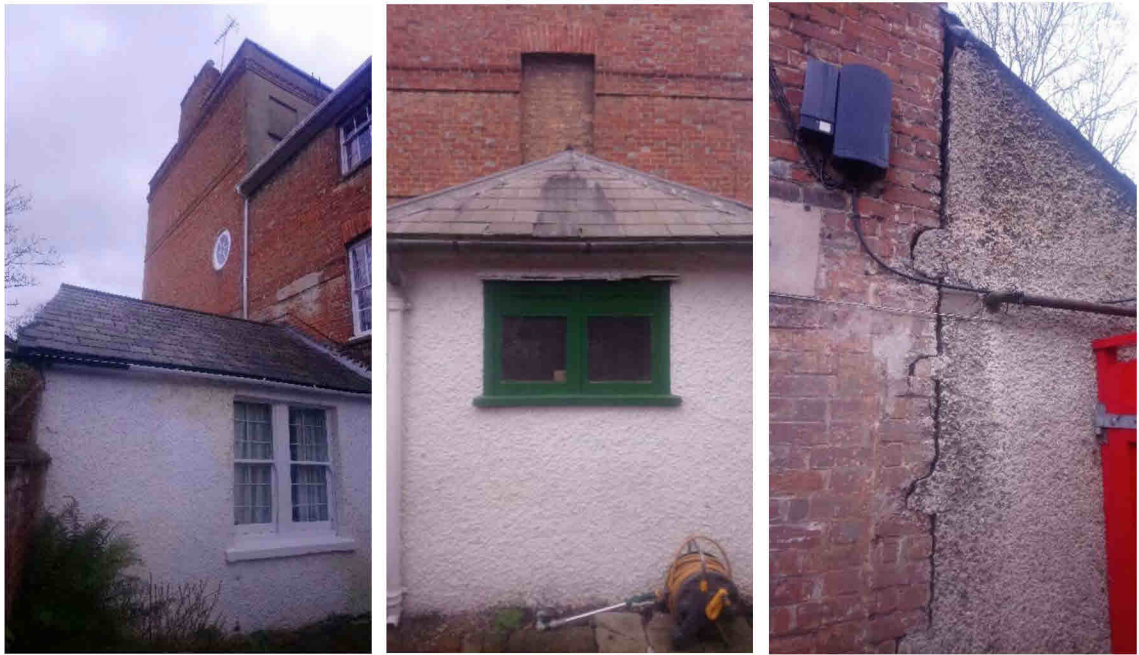
B5, north elevation with single storey 'extensions' (L & C) and crack between main house and extension on western elevation (R)
