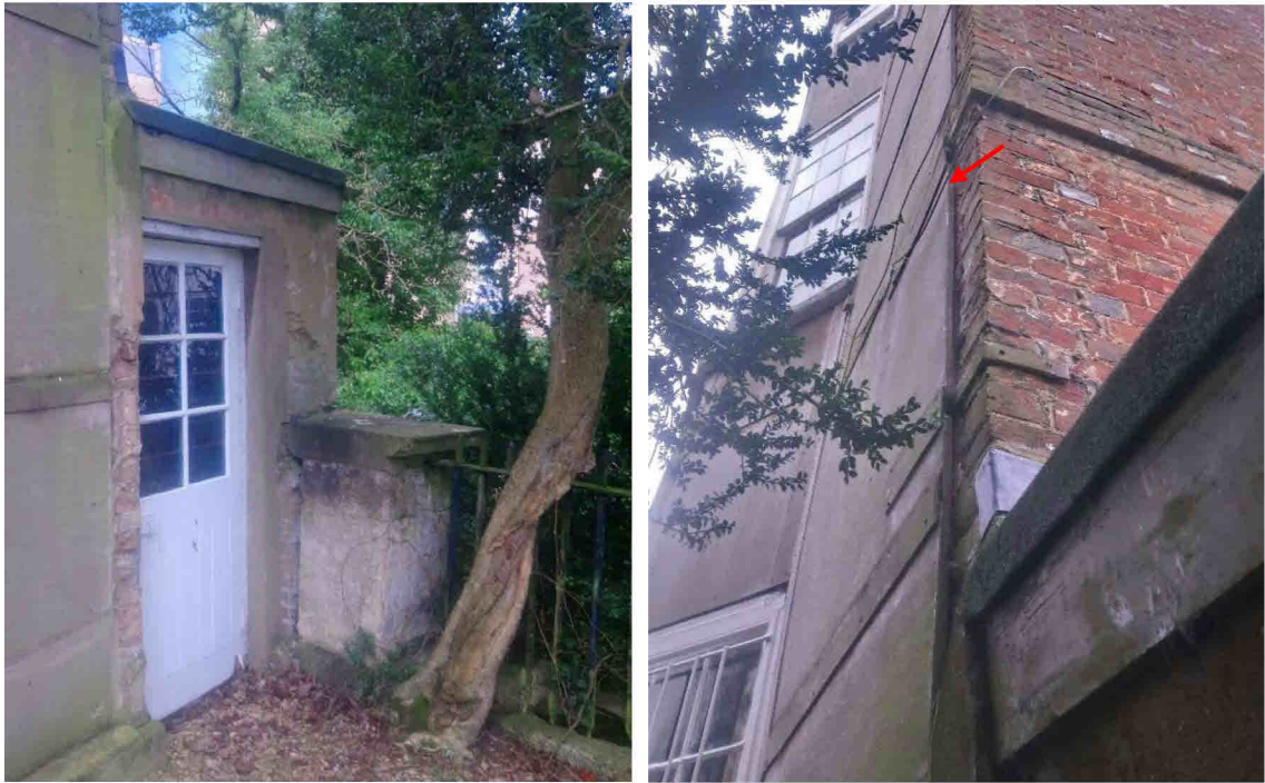
B5, eastern end of single storey extension on north side of building (L) and gaps behind plywood cladding, east elevation (R)
