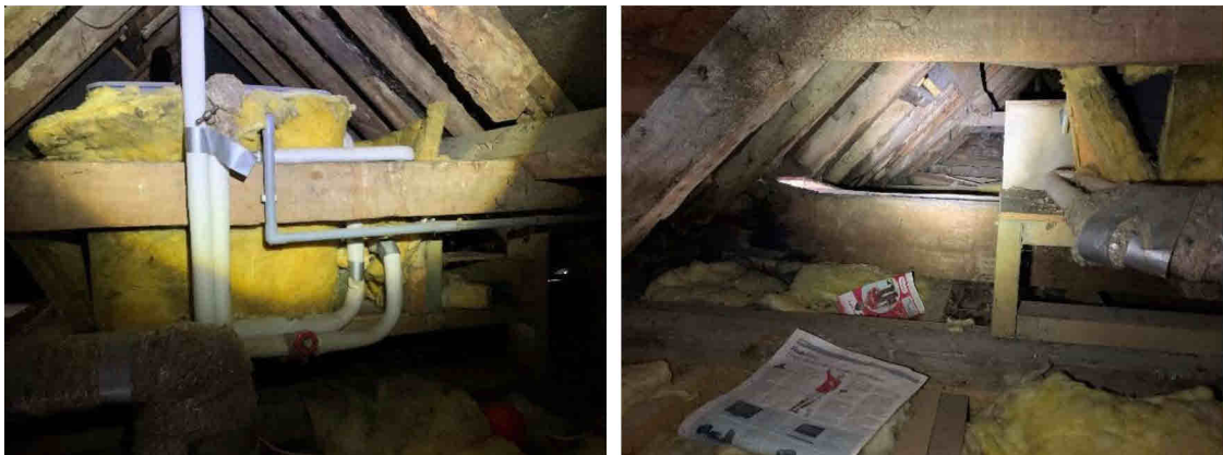
Eastern end of B5's roof void showing large water tank occupying most of the space
