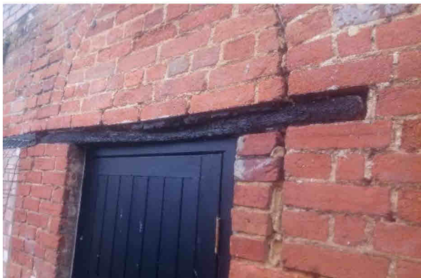
B2, cracks/gaps around lintel
