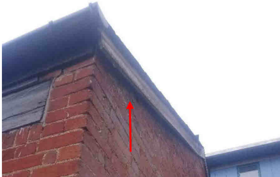
B1 gap under barge board
