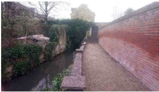
River Thames tributary which enters site via a culvert under the Abingdon Road, traverses then exits via culvert under building B5
