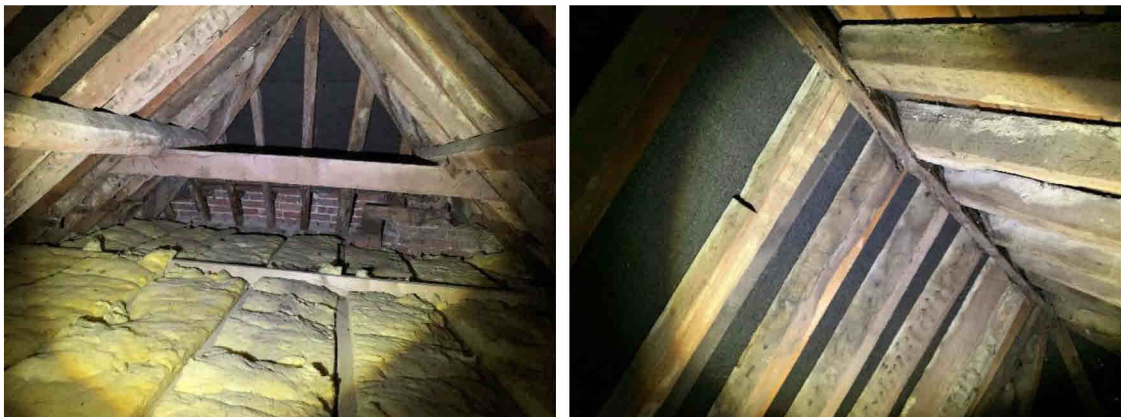
Western end of B5's roof void showing showing exposed timbers and sarking in good condition
